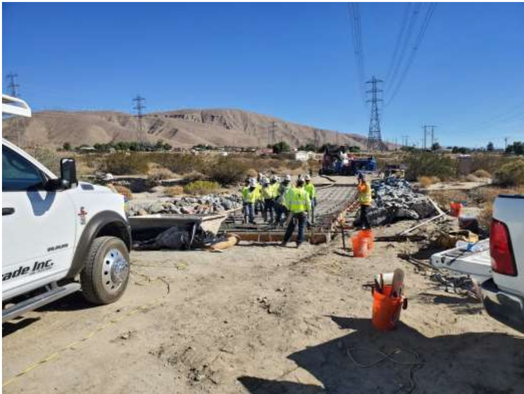
Photo 5 – Wet crossing installation on access road to Construction Area 6N41, Segment 6 (November 19, 2020).
