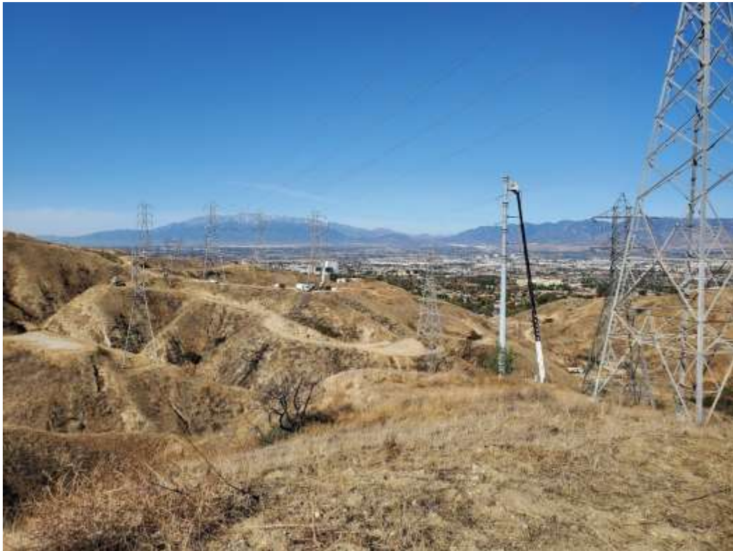
Photo 2 – Wire stringing activities at Construction Areas 2N01 and 3X65, Segments 2 and 3 (January 6, 2021).
