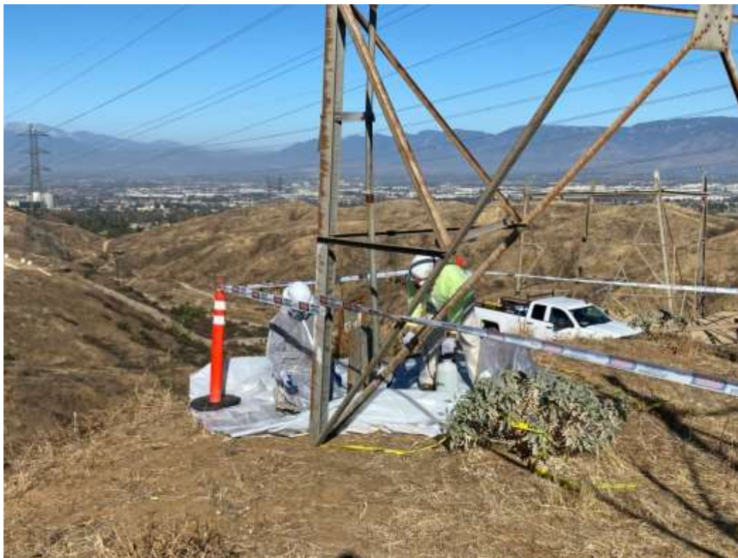
Photo 4 – Asbestos abatement at Construction Area 3X63, Segment 3 (January 4, 2021) (Photo courtesy of SCE).
