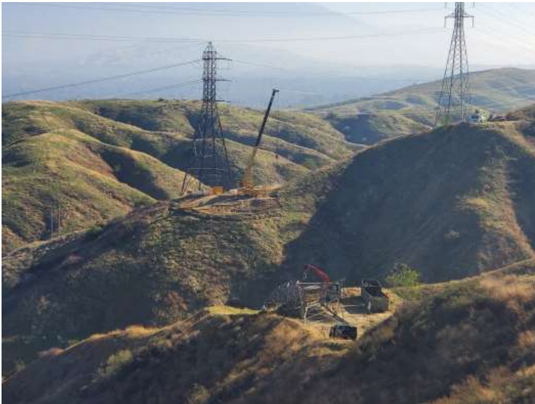
Photo 3 – Foundation installation activities at Construction Area 3X65 and tower wreck-out at Construction Area M3-T1, Segment 3 (February 4, 2021).
