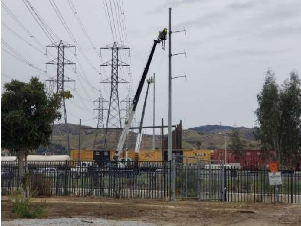
Photo 1 – Shoofly wire wreck-out activities at Construction Areas 1X10 through 1X11 (SF110 through SF111), Segment 1 (February 1, 2021).
