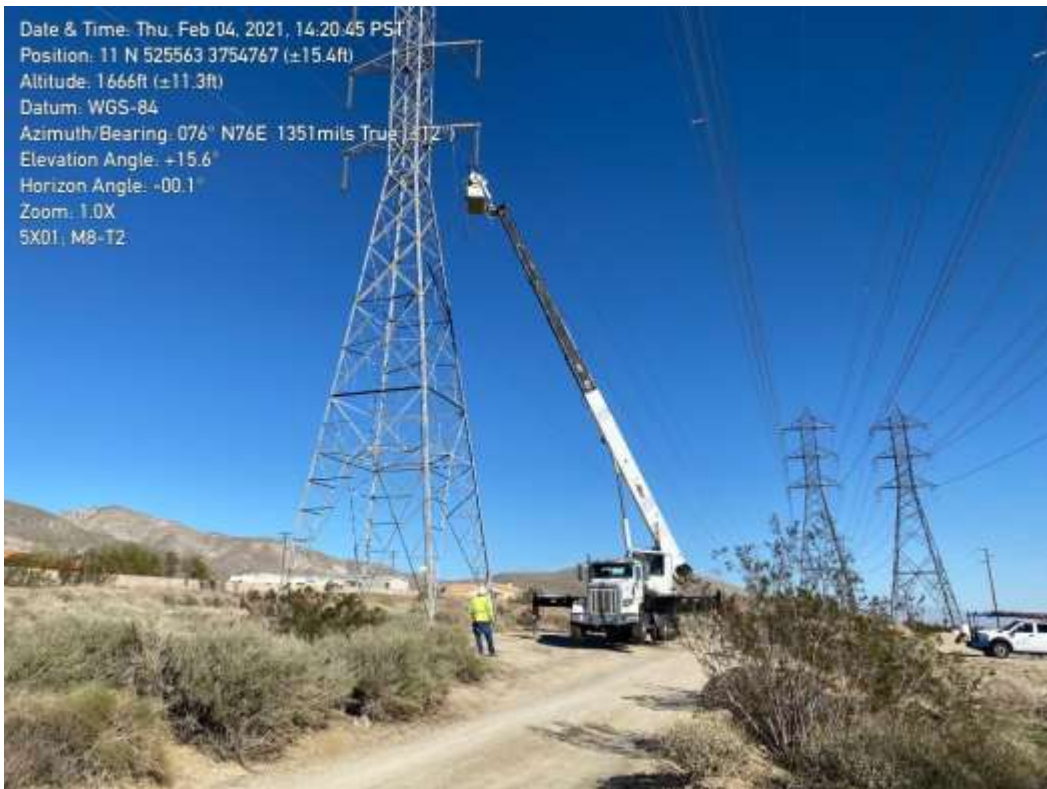
Photo 5 – Wire wreck-out activities at Construction Area 5X01, Segment 5 (Photo courtesy of SCE) (February 4, 2021).
