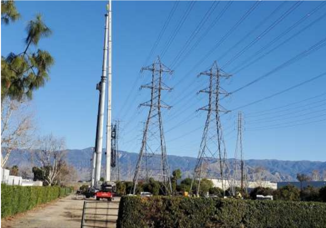
Photo 1 – Shoofly tower wreck-out at Construction 1X19 (SF121), Segment 1 (February 18, 2021).
