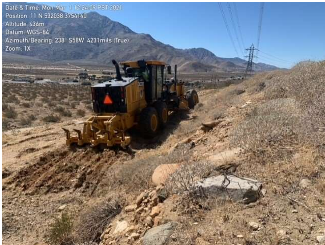
Photo 6 – Site scarification at Construction Area 6S29, Segment 6 (Photo courtesy of SCE) (March 1, 2021).
