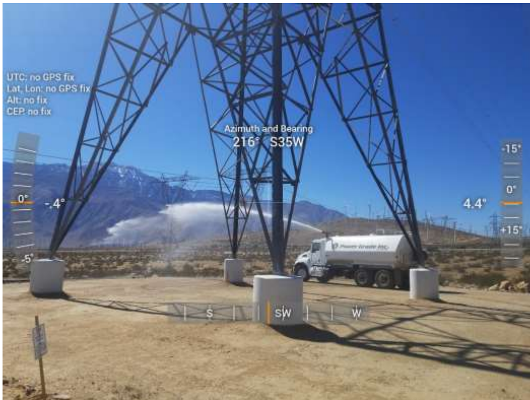
Photo 5 – Hydroseed watering at Construction Area 6X13, Segment 6 (Photo courtesy of SCE) (March 2, 2021).
