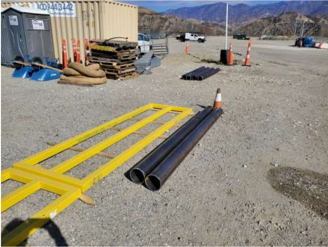
Photo 1 – Uncapped and uncovered construction pipes at the Match MY (March 3, 2021).
