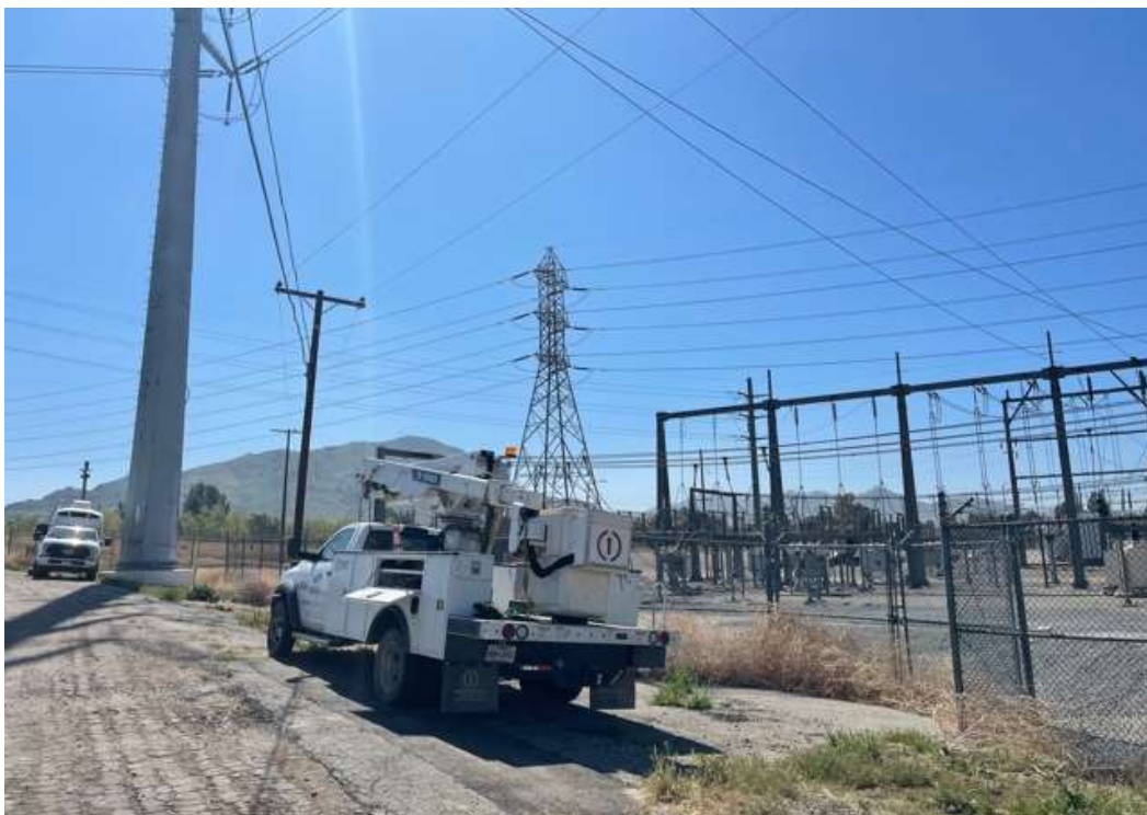
Photo 2 – Fiber splicing activities at Construction Area 2N36, Segment 2 (April 7, 2021) (Photo courtesy of SCE).
