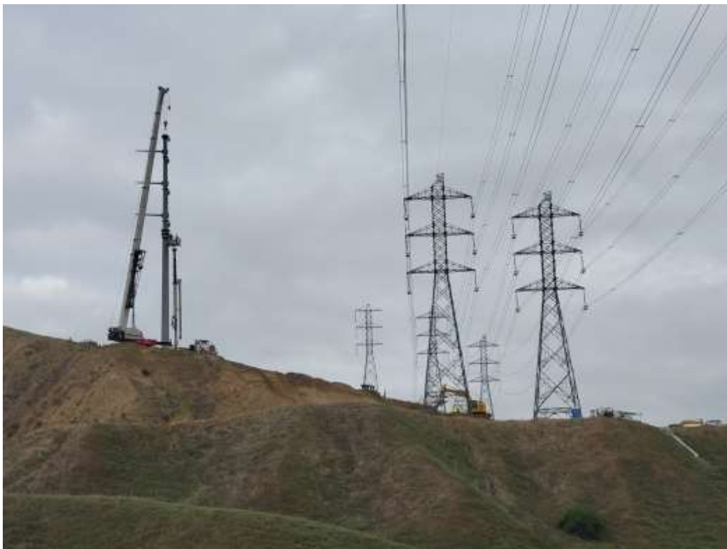
Photo 4 – Tower wreck-out and tower pad re-contouring at Construction Area 3X31, Segment 3 (April 14, 2021).
