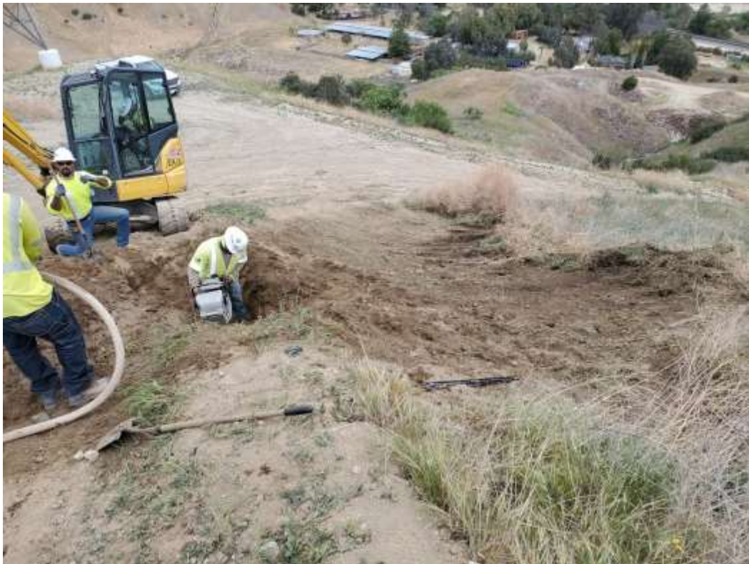
Photo 3 – MAC drain vegetation clearing and installation at Construction Area 3X37, Segment 3 (April 21, 2021).
