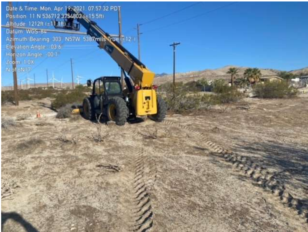
Photo 6 – Forklift staged outside of approved Construction Area WA-6-6N17-MPR-35, Segment 6 (April 19, 2021) (Photo courtesy of SCE).
