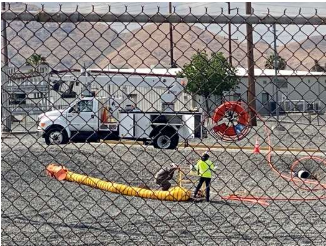
Photo 2 – Fiber optic installation at the Vista Substation (April 27, 2021) (Photo courtesy of SCE).
