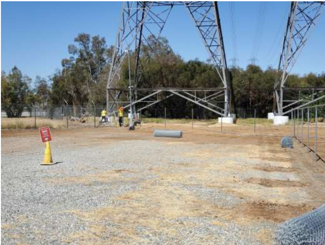
Photo 7 – Fence installation at Construction Area 4X44 (within approved vertical nest buffer reduction), Segment 4 (April 28, 2021).
