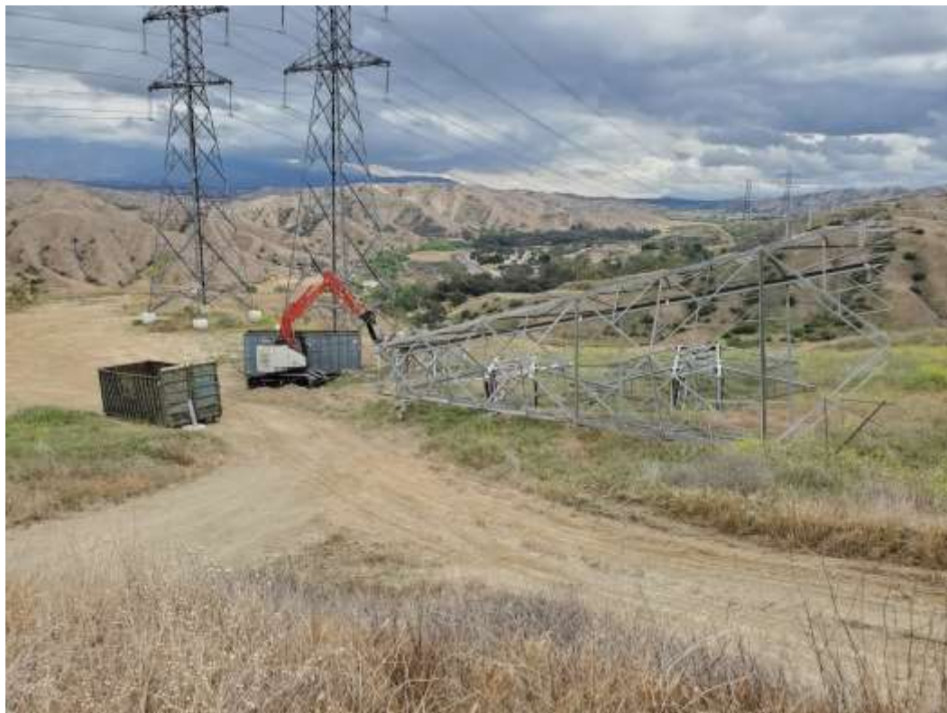
Photo 4 – Tower shearing at Construction Area 3X38, Segment 3 (April 26, 2021).
