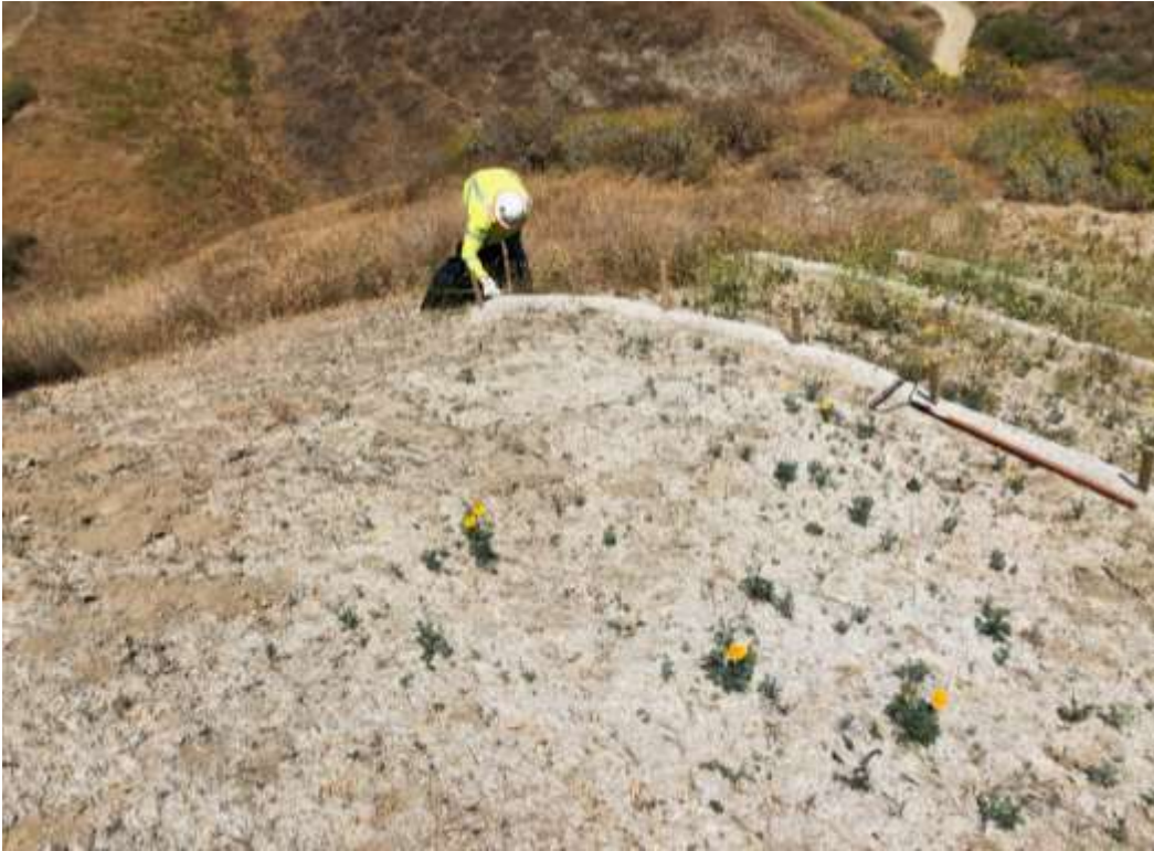
Photo 1 – Hand weed removal at Construction Area 2N10, Segment 2 (May 13, 2021) (Photo courtesy of SCE).
