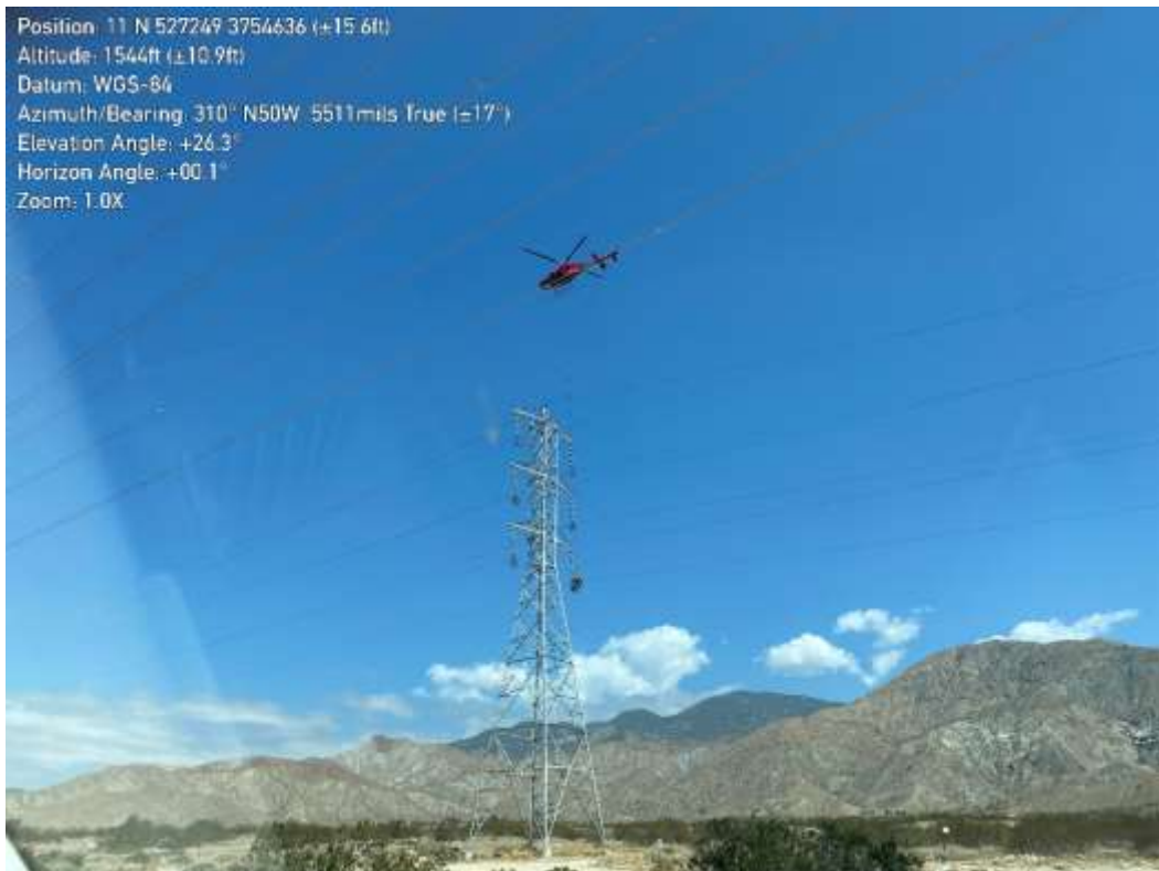
Photo 6 –Helicopter activities incident at Construction Area 6X44, Segment 6 (May 22, 2021) (Photo courtesy of SCE).
