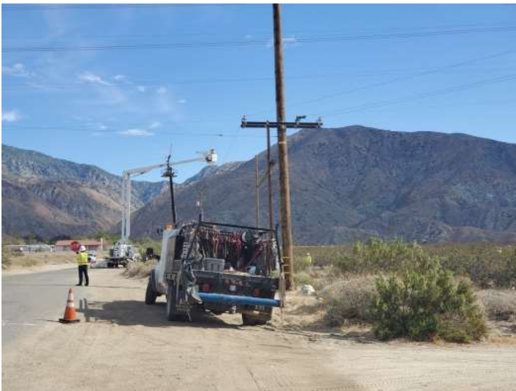
Photo 4 – Wire wreck-out activities between Construction Areas 5X01 and 6X48, Segments 5 and 6 (May 26, 2021).
