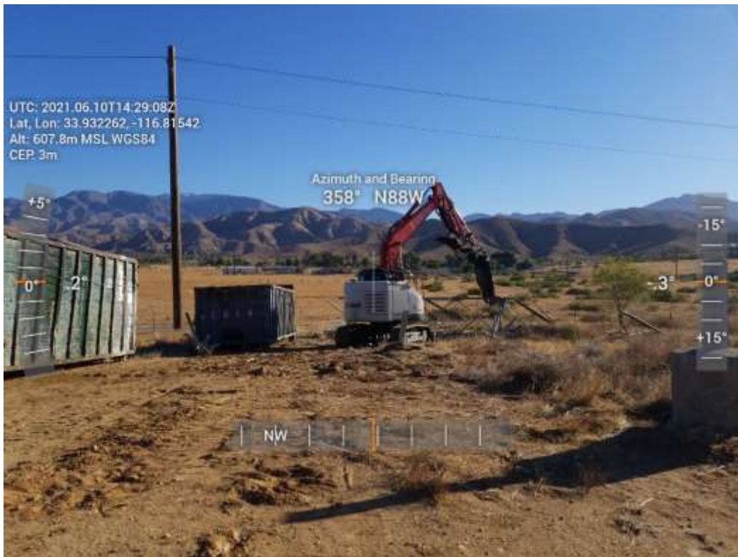
Photo 4 – Tower shearing activities at Construction Area M13-T2, Segment 5 (June 10, 2021) (Photo courtesy of SCE).
