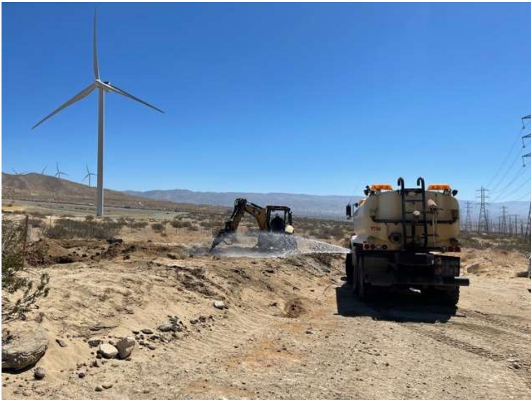
Photo 5 – Foundation wreck-out at Construction Area M62-T4, Segment 6 (June 8, 2021) (Photo courtesy of SCE).
