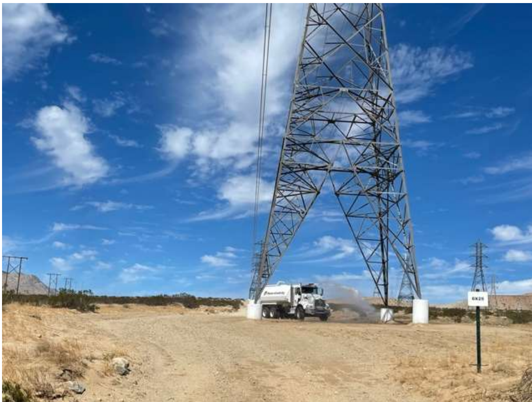
Photo 6 – Hydroseed watering at Construction Area 6S25, Segment 6 (June 9, 2021) (Photo courtesy of SCE).
