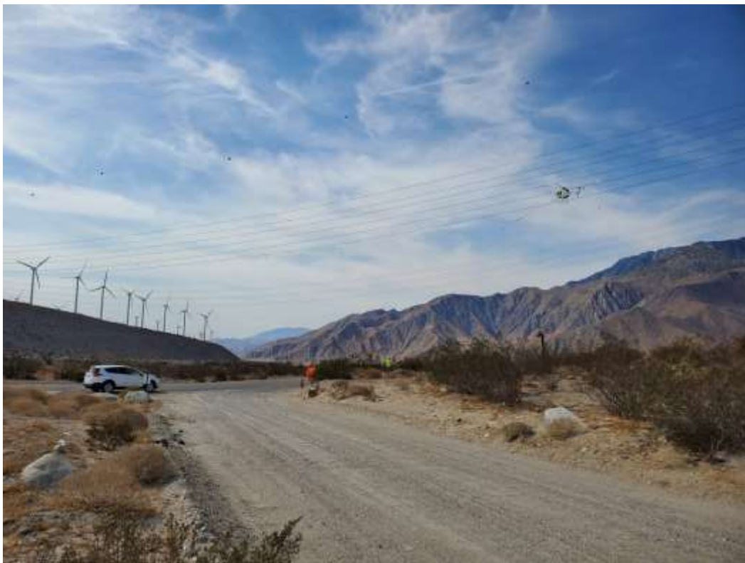
Photo 6 – Helicopter wire wreck-out activities and traffic control at Construction Area 6N28, Segment 6 (June 15, 2021).
