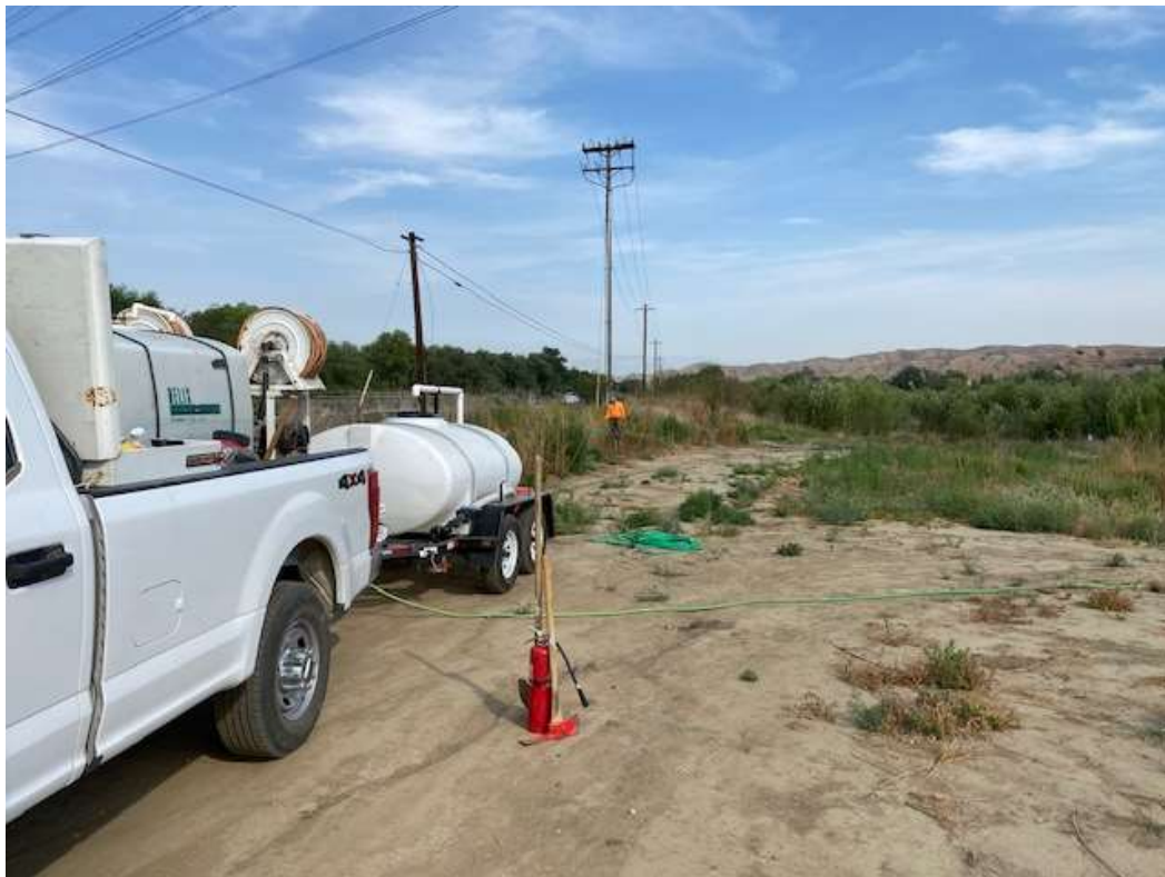
Photo 4 – Restoration monitoring at Construction Area 4N63, Segment 4 (June 16, 2021) (Photo courtesy of SCE).
