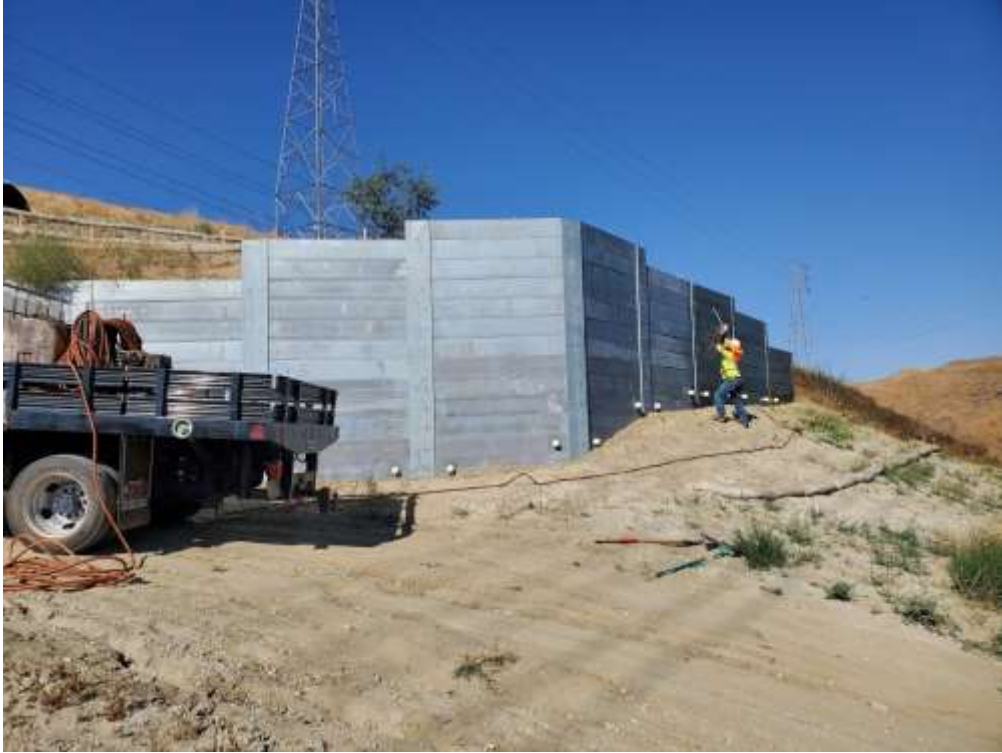
Photo 1 – Natina application to soldier pile wall at Construction Area 2N11, Segment 2 (June 21, 2021).
