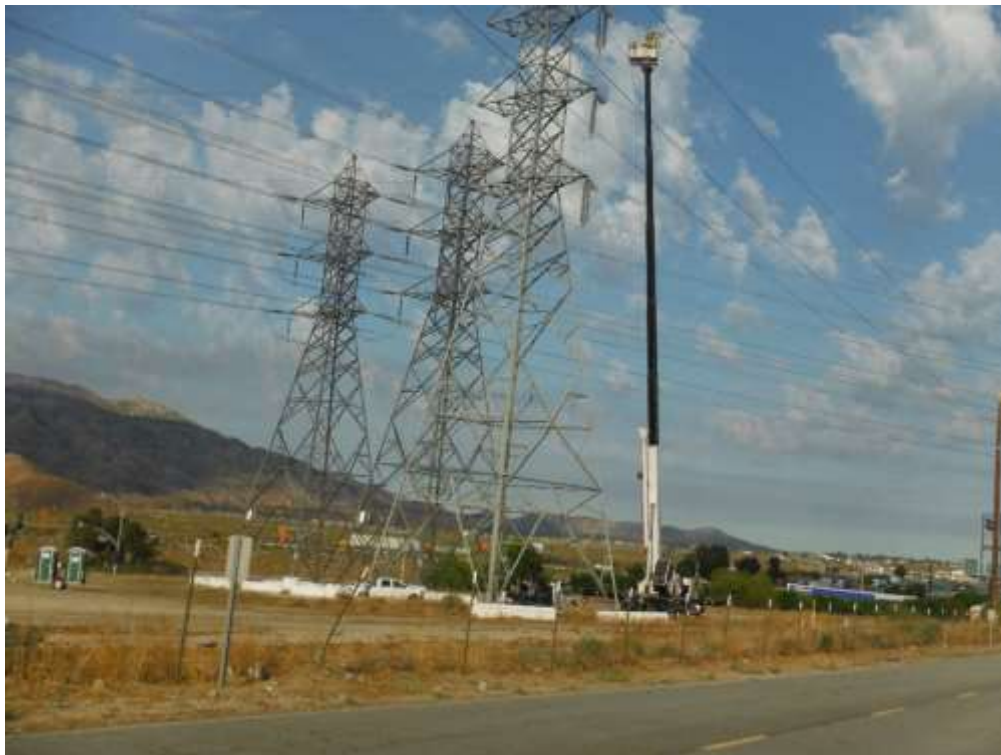
Photo 4 – Wire wreck-out activities at Construction Area 5X29, Segment 5 (June 24, 2021) (Photo courtesy of SCE).
