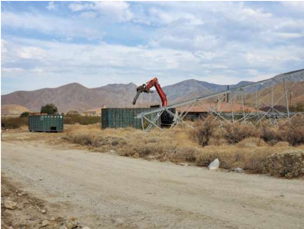
Photo 4 – Tower shearing at Construction Area 5X01, Segment 5 (June 29, 2021).
