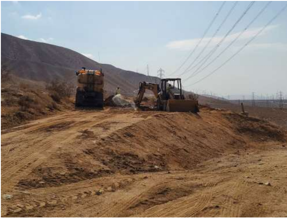
Photo 5 – Foundation wreck-out at Construction Area 6N35, Segment 6 (July 12, 2021).
