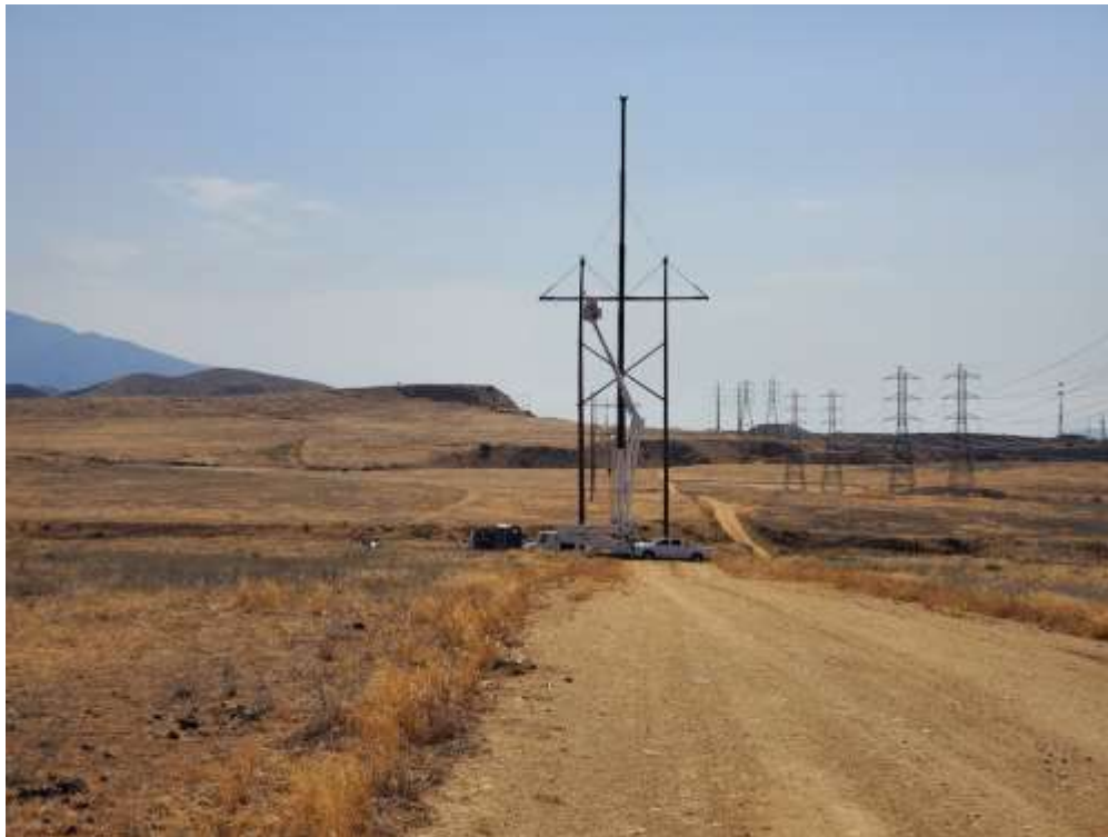
Photo 4 – H-frame wreck-out at Construction Area 4X09, Segment 4 (July 12, 2021).
