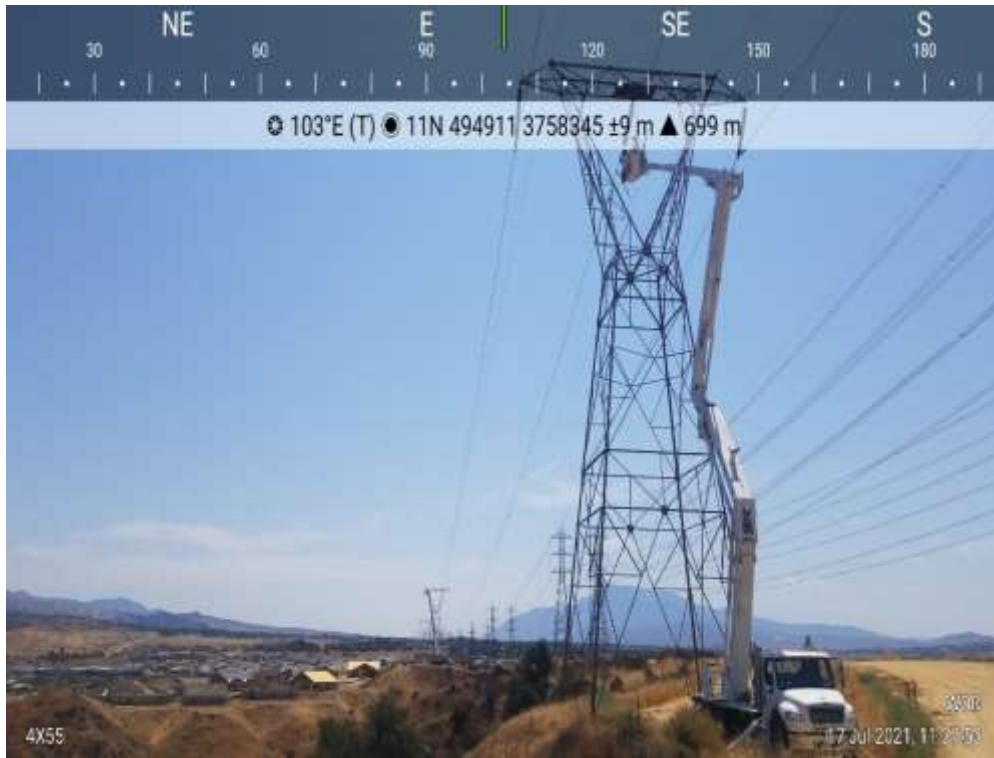
Photo 3 – Wire wreck-out activities at Construction Area 4X55, Segment 4 (July 17, 2021) (Photo courtesy of SCE).
