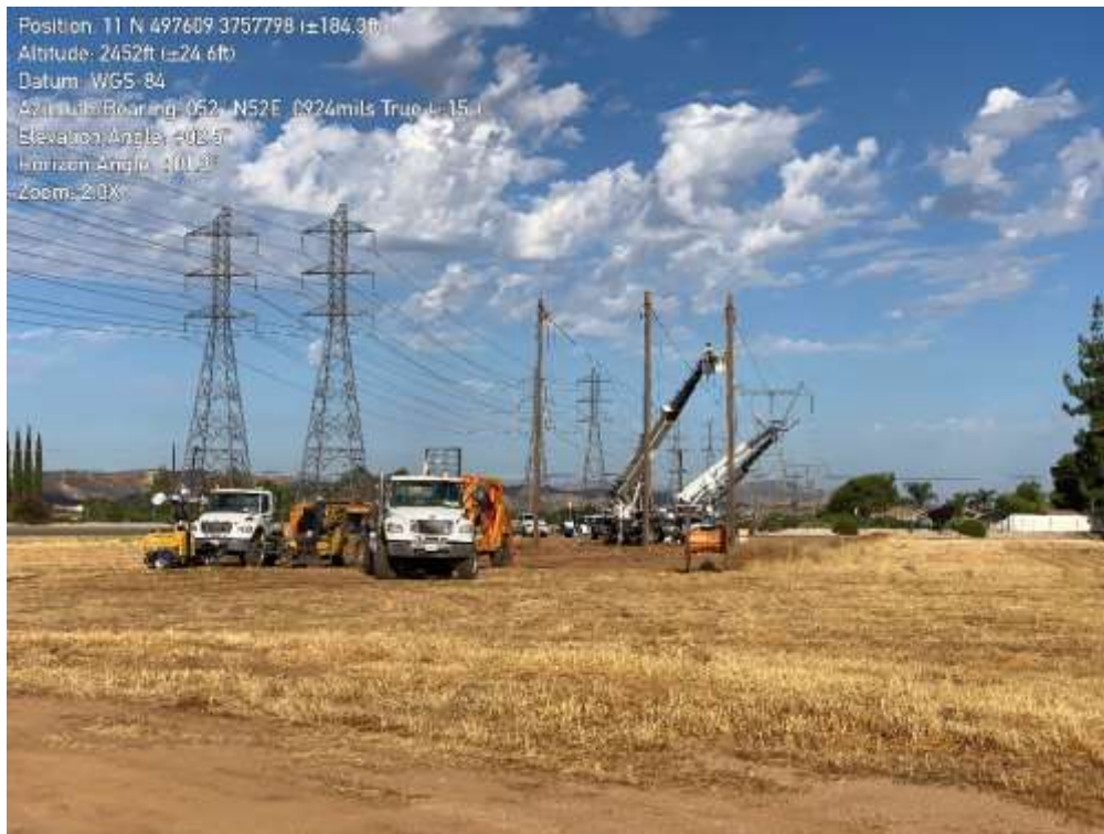
Photo 3 – Wire wreck-out activities at Construction Area WSS-4X45-4X46, Segment 4 (July 19, 2021) (Photo courtesy of SCE).
