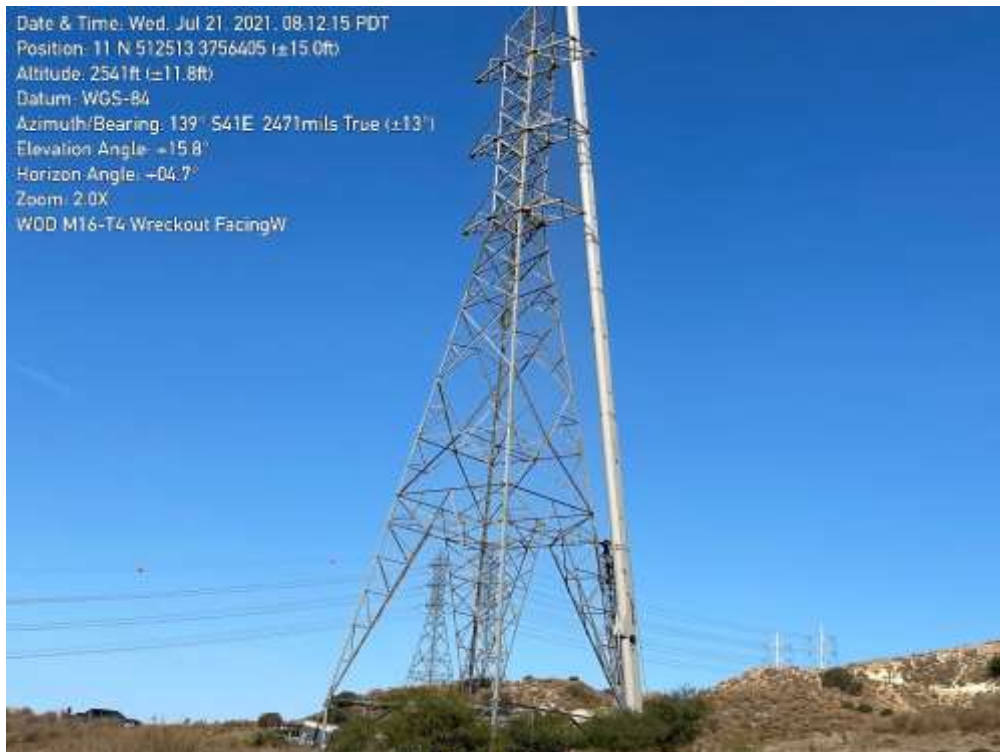
Photo 4 – Tower wreck-out at Construction Area M76-T4, Segment 5 (July 21, 2021) (Photo courtesy of SCE).
