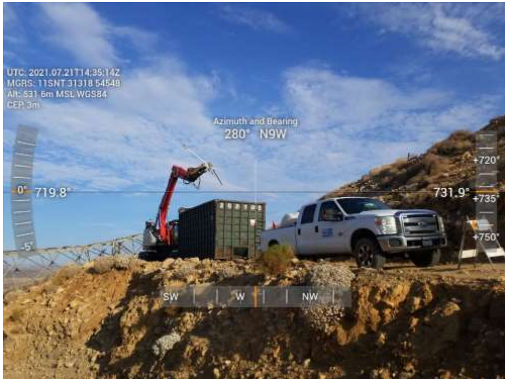
Photo 6 – Tower shearing at Construction Area 6N31, Segment 6 (July 21, 2021) (Photo courtesy of SCE).
