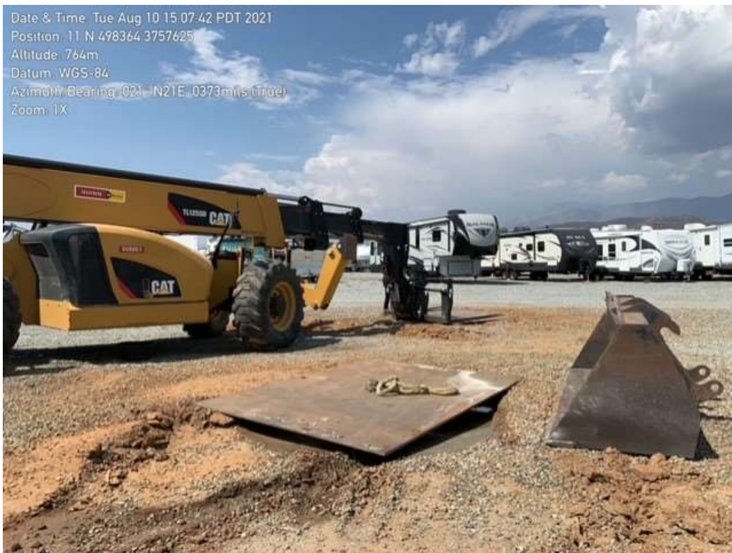
Photo 4 – Foundation slurry backfill at Construction Area 4X44-1, Segment 4 (August 10, 2021) (Photo courtesy of SCE).
