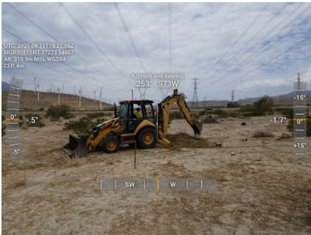
Photo 6 – Anchor removal at Construction Area 6S15, Segment 6 (August 11, 2021) (Photo courtesy of SCE).
