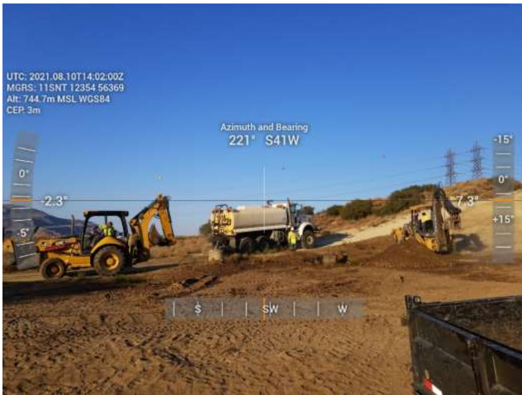
Photo 5 – Foundation wreck-out at Construction Area M76-T4, Segment 5 (August 10, 2021) (Photo courtesy of SCE).
