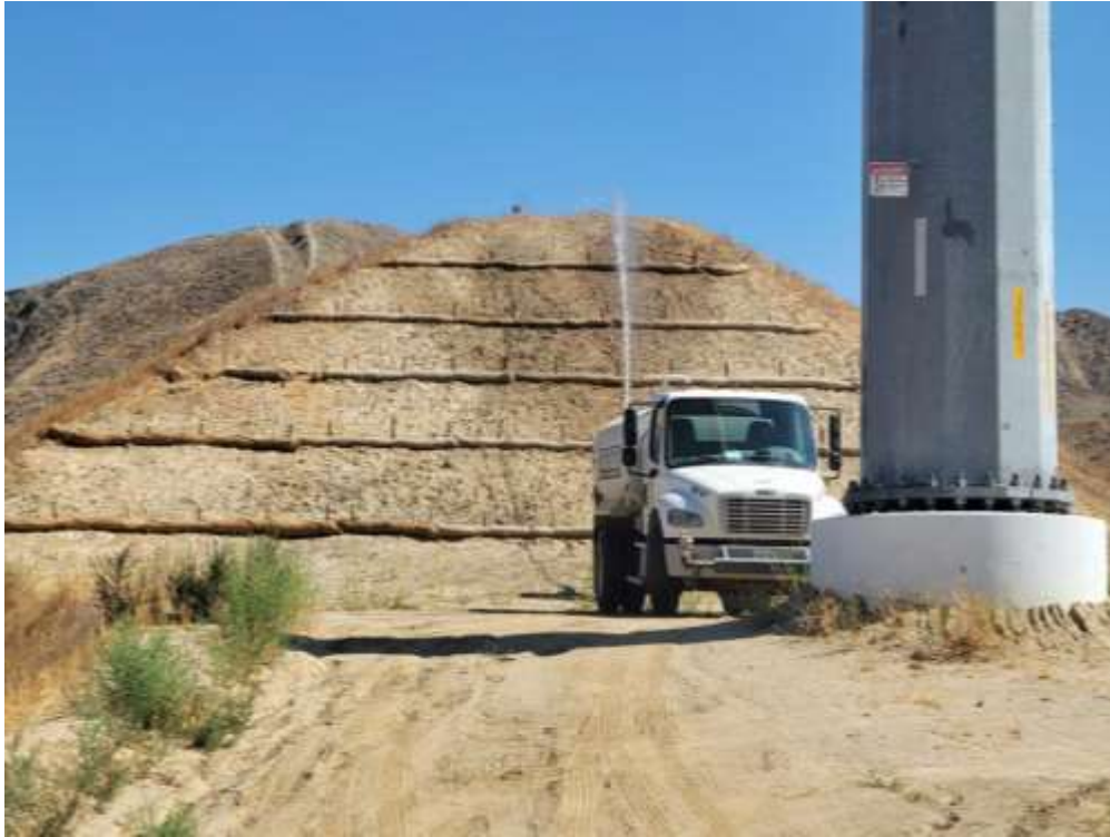
Photo 1 – Hydroseed watering at Construction Area 2N15, Segment 2 (August 26, 2021) (Photo courtesy of SCE).
