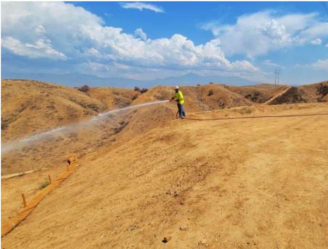
Photo 3 – Hydroseed watering at Construction Area 3X64, Segment 3 (September 9, 2021) (Photo courtesy of SCE).
