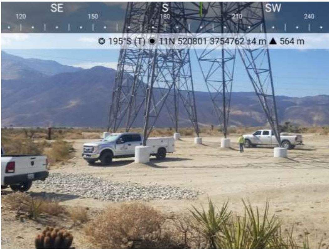
Photo 5 – Foundation punch-list activities at Construction Area 5X16, Segment 5 (September 9, 2021) (Photo courtesy of SCE).
