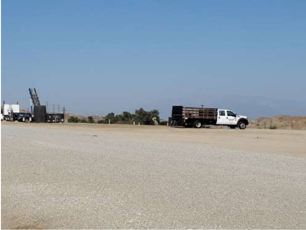
Photo 1 – Clean-up and soil export of the equipment wash-out and fuel containment areas at the Poultry MY (September 21, 2021).
