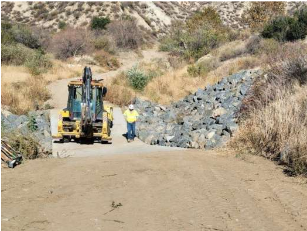
Photo 4 – Rip-rap replacement at Construction Area 4X04-SE, Segment 4 (November 3, 2021) (Photo courtesy of SCE).
