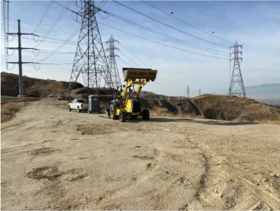
Photo 1 – Site decompaction and hydroseed preparation at Construction Area 2N01, Segment 2 (December 6, 2021) (Photo courtesy of SCE).
