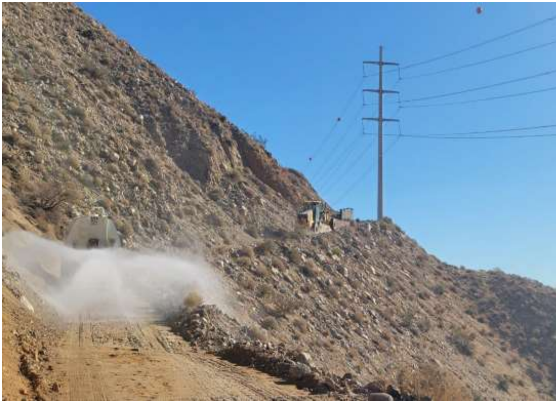
Photo 6 – Access road grading to Construction Area 6N31, Segment 6 (November 29, 2021) (Photo courtesy of SCE).
