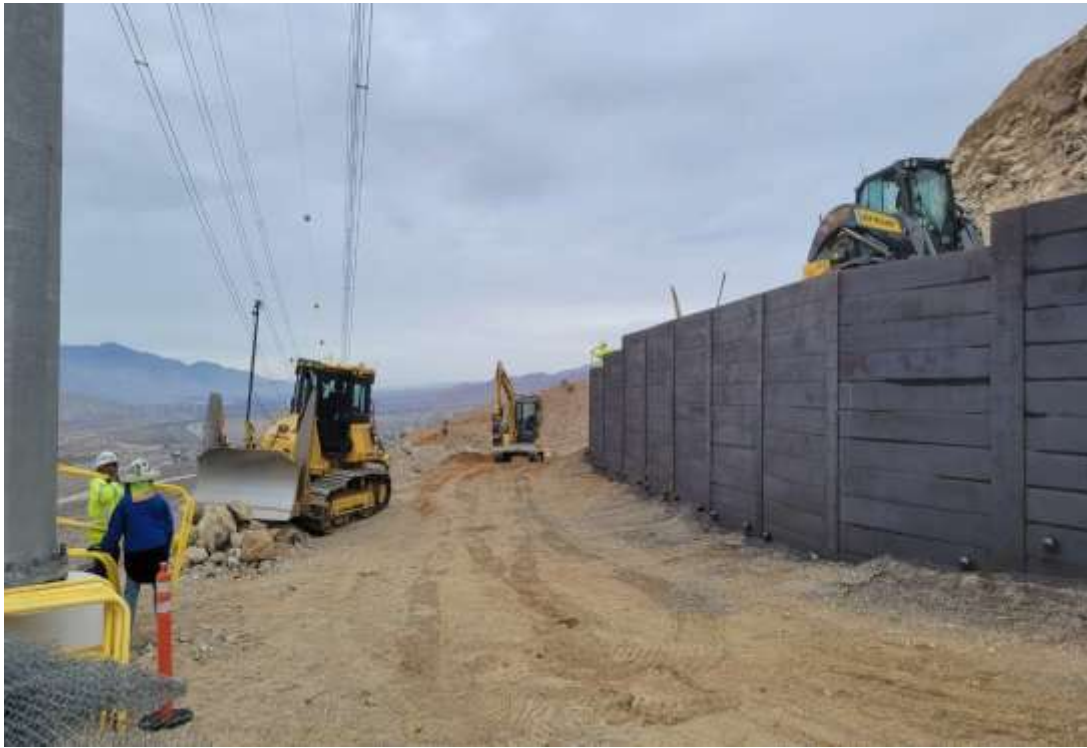
Photo 5 – Site restoration and wall backfilling at Construction Area 6N30, Segment 6 (December 7, 2021) (Photo courtesy of SCE).
