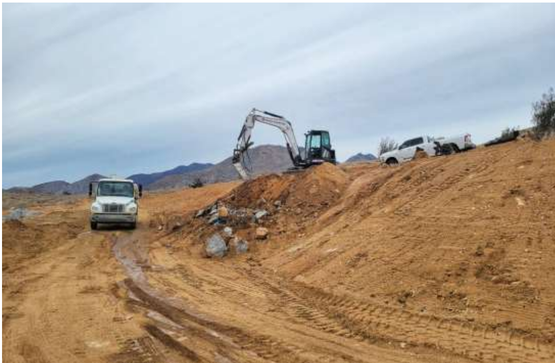
Photo 4 – Subgrade foundation excavation at Construction Area 6N35, Segment 6 (December 10, 2021) (Photo courtesy of SCE).
