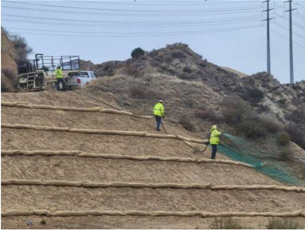
Photo 1 – Hydroseed application at Construction Area 4X04-SE-1, Segment 4 (December 21, 2021) (Photo courtesy of SCE).
