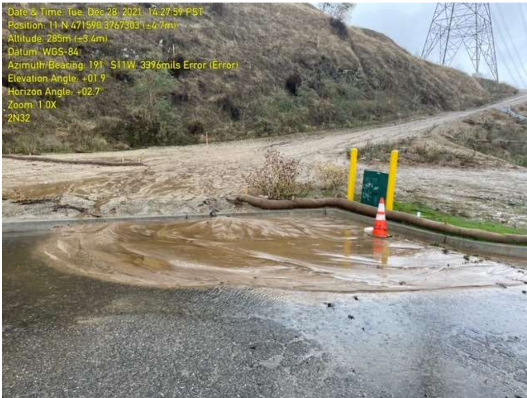
Photo 6 – Erosion issues to be addressed at Construction Area 2N32, Segment 2 (December 28, 2021) (Photo courtesy of SCE).
