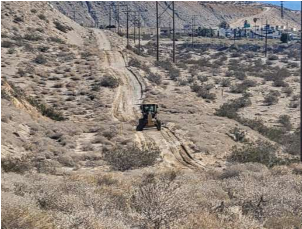
Photo 5 – Access road maintenance at Construction Area 6N29, Segment 6 (December 20, 2021) (Photo courtesy of SCE).
