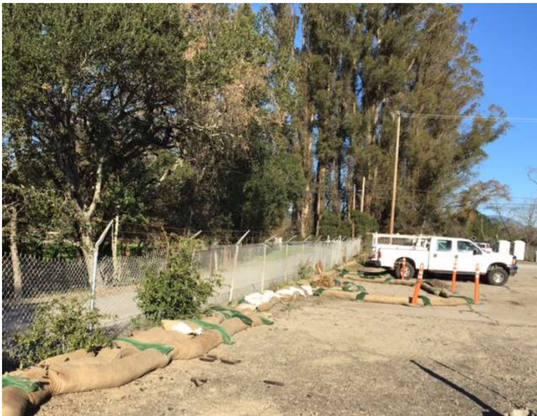
Figure 4 – Additional BMPs were installed on the northern side of the substation site, December 22, 2016.
