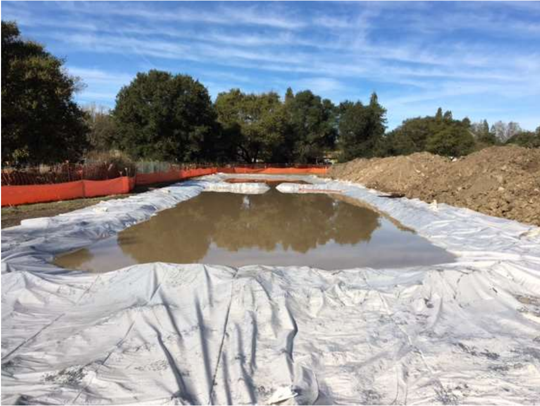
Figure 1 – A second storm water retention pond was constructed on the western side of the substation site adjacent to the first pond, December 20, 2016.
