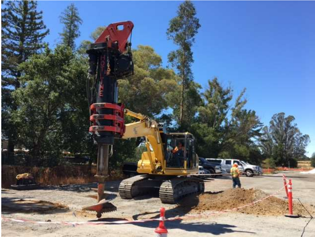
Figure 1 – Drilling pier holes for perimeter wall foundation on east side of site – view west-southwest, July 26, 2017.
