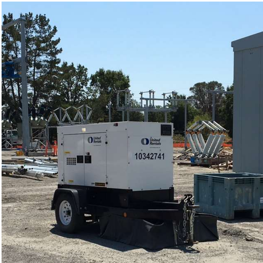
Figure 3 – Generator in need of additional secondary containment – view southwest, August 1, 2017.
