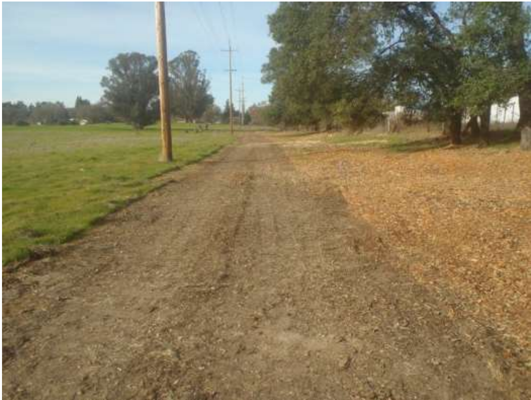
Figure 5 – Access road to TSP where mats were removed the previous week – view north, December 27, 2017. Photo courtesy of PG&E.
