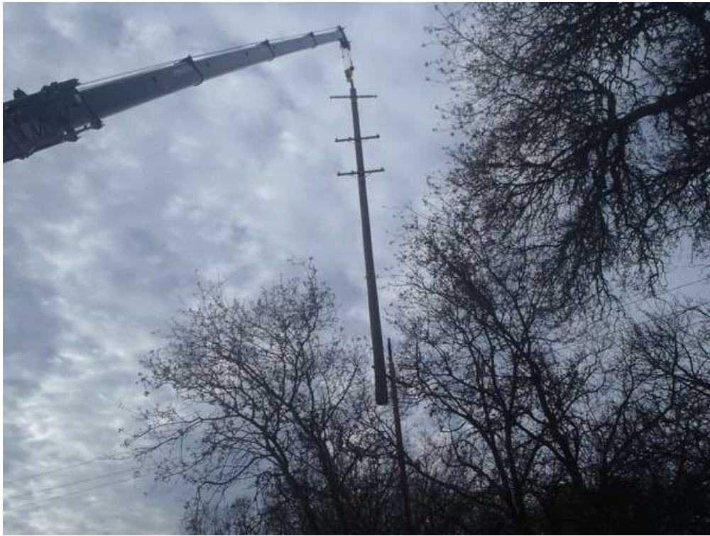
Figure 3 – Crane lifting pole into place over trees – view west, December 19, 2017. Photo courtesy of PG&E.
