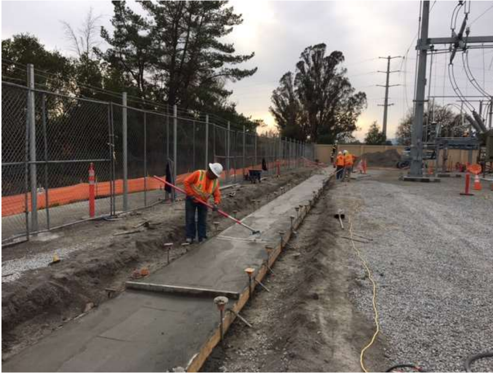
Figure 1 – Crews working on a V-ditch on the south side of the Substation – view west, December 19, 2017.
