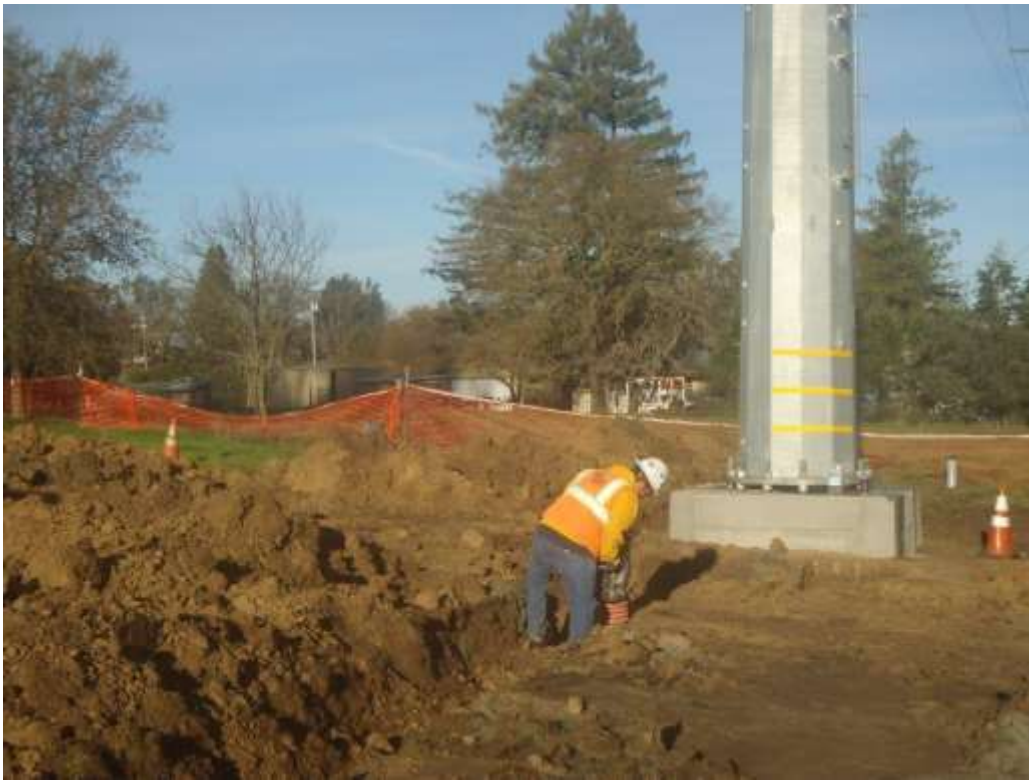
Figure 7 – Backfilling and compacting conduit trench to TSP – view north, December 28, 2017. Photo courtesy of PG&E.
