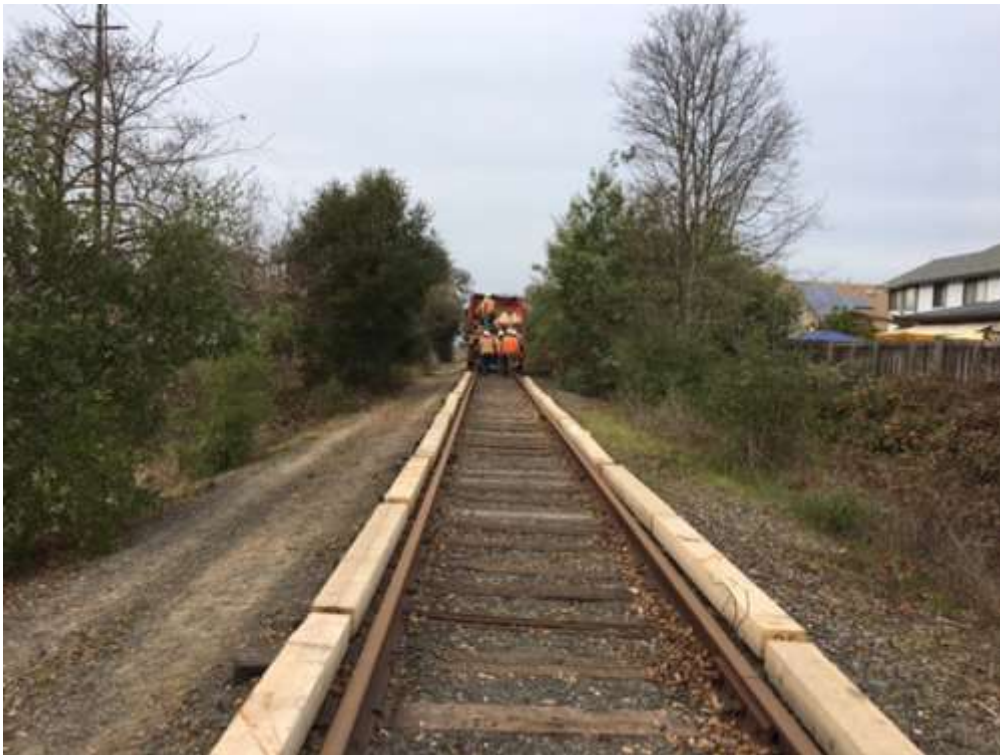
Figure 4 – Crews picking up wood beams used to drive cranes on over railroad tracks – view north, December 19, 2017.
