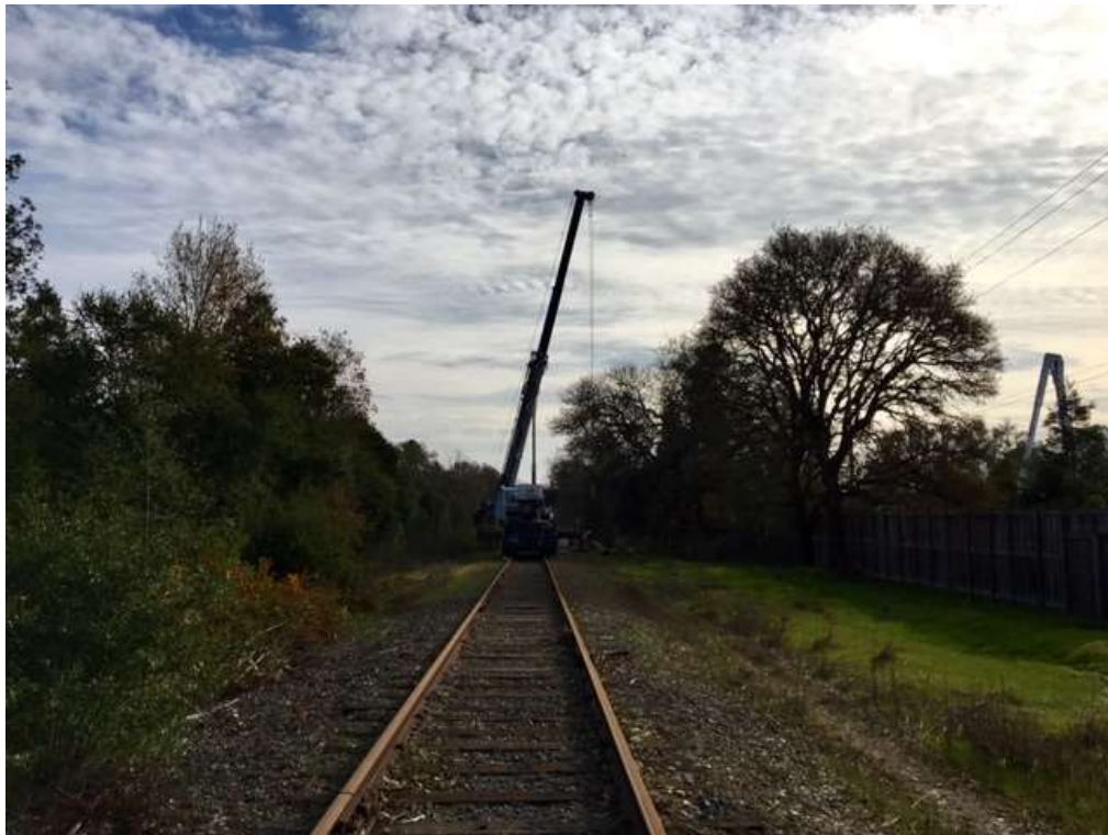
Figure 2 – Crews preparing pole for replacement with crane along the railroad – view south, December 19, 2017.
