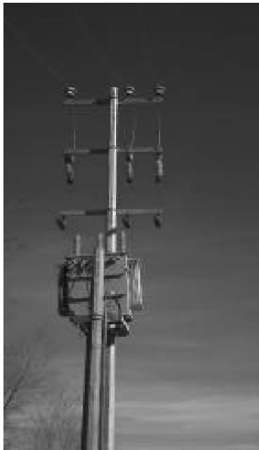
Photo by Cynthia Melcher Photo 3. Concrete pole associated with raptor electrocutions in San Pedro, Mexico.
