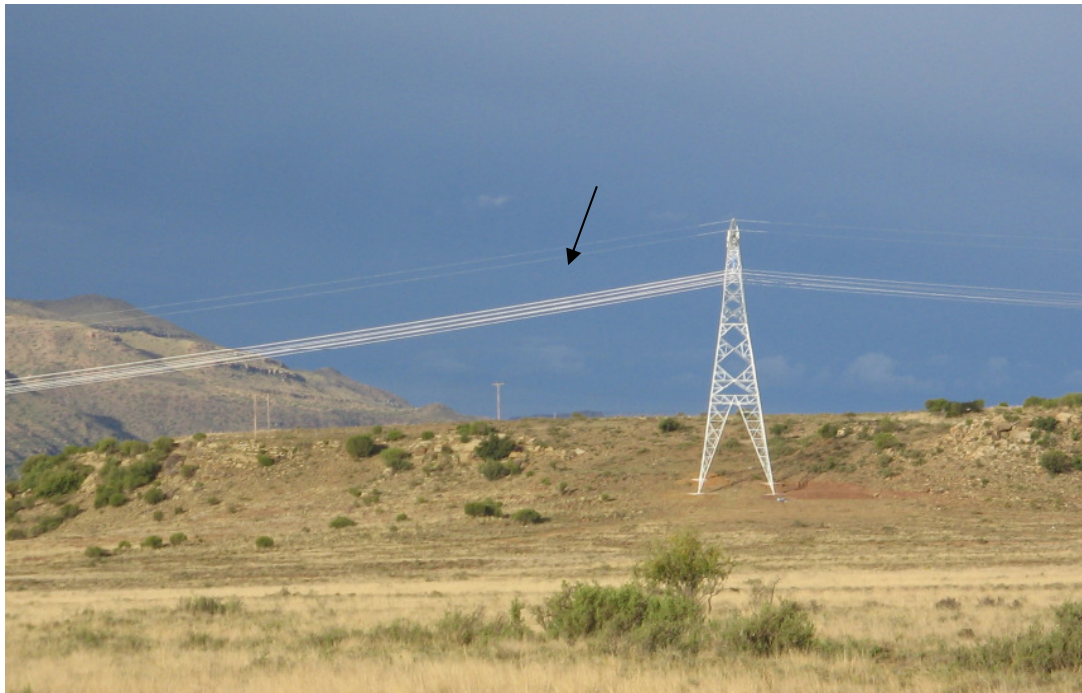
Figure 16. A 400 kV line, with all conductor wires in the same horizontal plane. This picture also demonstrates the almost invisible thin earth wire (black arrow) in top (Photo: EWT-WEP).
