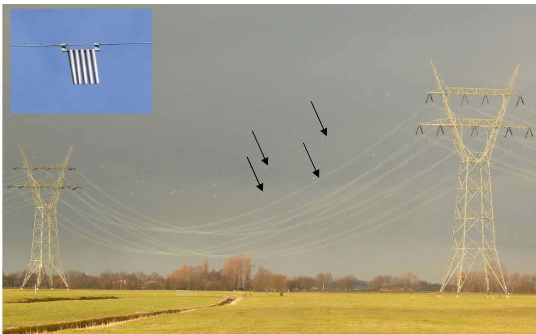
Figure 20. High tension (150 kV) power line in the Netherlands with bird flappers (see arrows) placed at regular intervals in both ground wires as bird flight diverters, see also Box 1 (Photo: Bureau Waardenburg).
