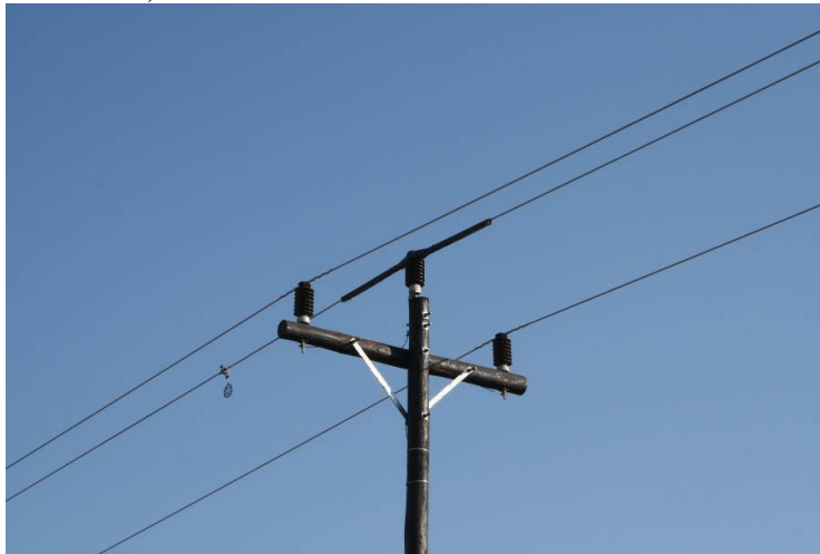
Figure 13. A 'Raptor Protector' used to insulate the centre conductor of a 22 kV pole structure making the distances between non-insulated conductors large enough for safe perching (Photo: EWT-WEP).
