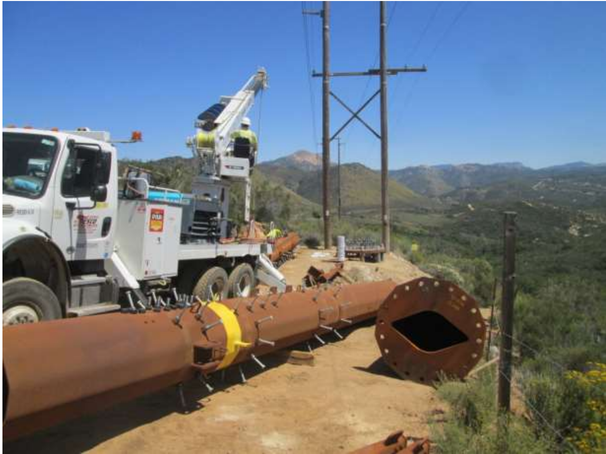
Photo 4: A construction crew observed framing steel replacement poles and preparing to set them at Pole Z272852 (TL625B).
