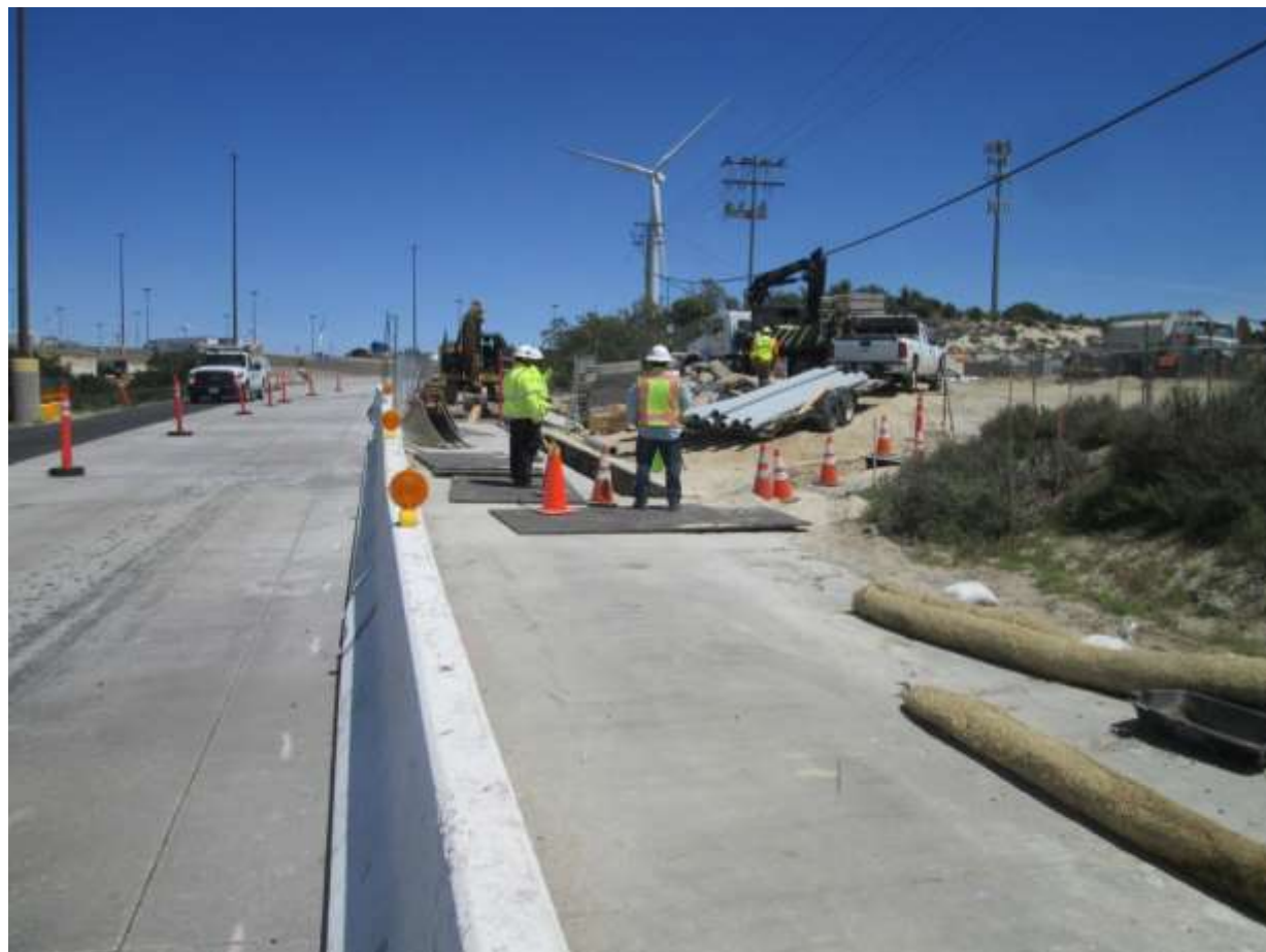
Photo 3: A construction crew observed trenching and laying conduit encasement piping at the Old Highway 80 jack-and-bore crossing (TL629E) near Crestwood Substation.
