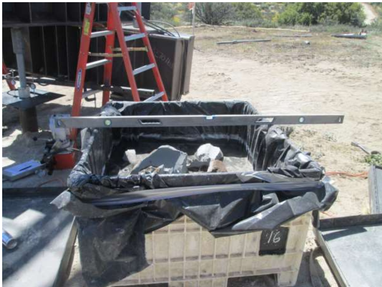
Photo 5: In accordance with APM HYD-1, concrete waste generated during micropile foundation construction at Pole Z44271 (TL6931) was cleaned up and disposed of in accordance with approved procedures.
