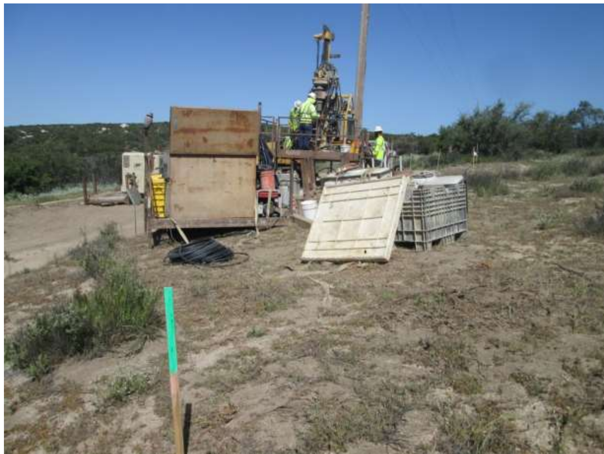
Photo 2: A construction crew observed drilling for a micropile foundation at Pole Z44248 (TL6931). The work activity was restricted to the delineated workspace (marked with green painted stakes) in accordance with MM BIO-1.
