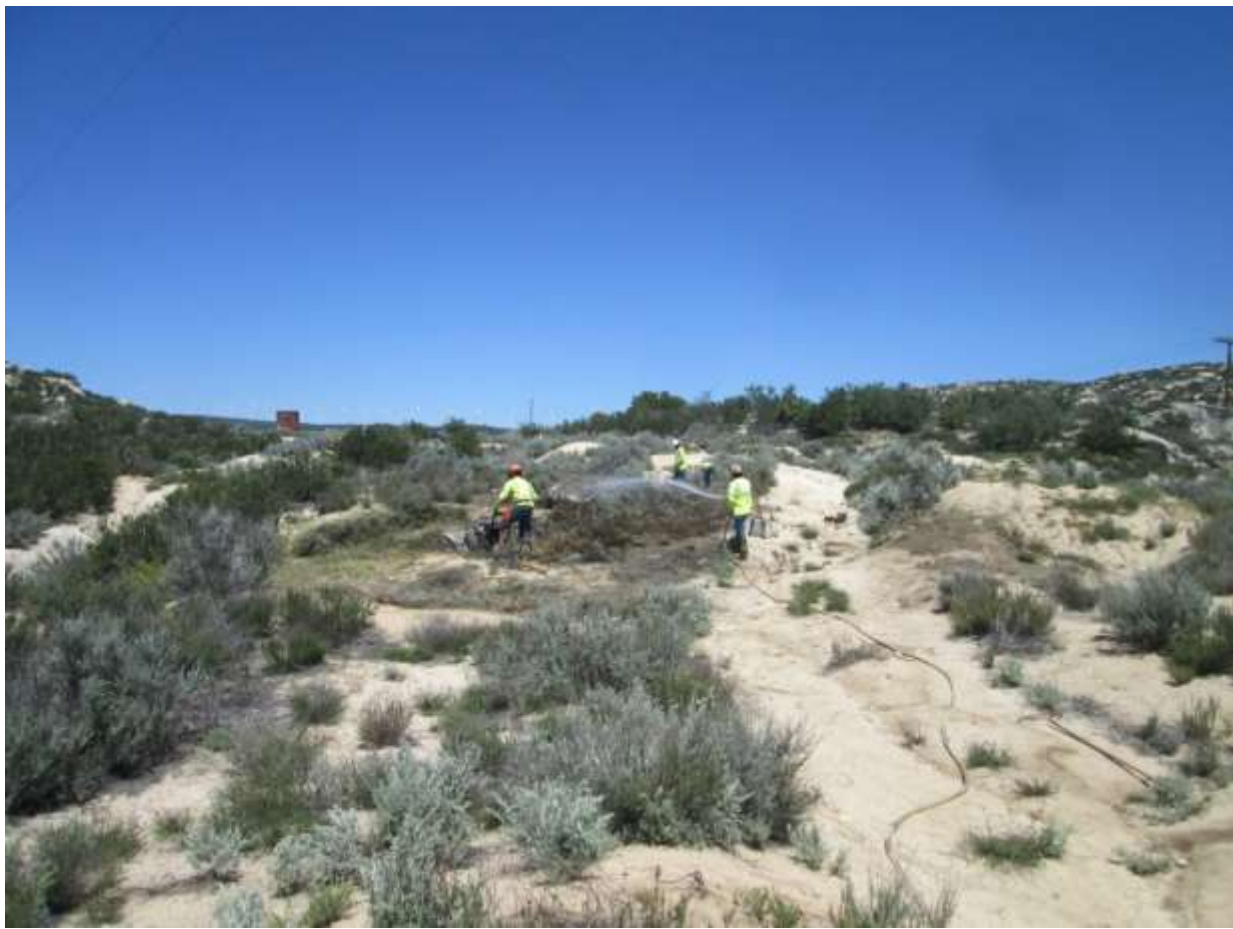
Photo 1: During vegetation clearing at the Pole Z44253 Stringing Site (TL6931), the construction crew pre-watered the work area and staged the prescribed fire tools were within 50 feet in accordance with the CFPPP, MM FF-1, APM HAZ-01, and APM HAZ-04.
