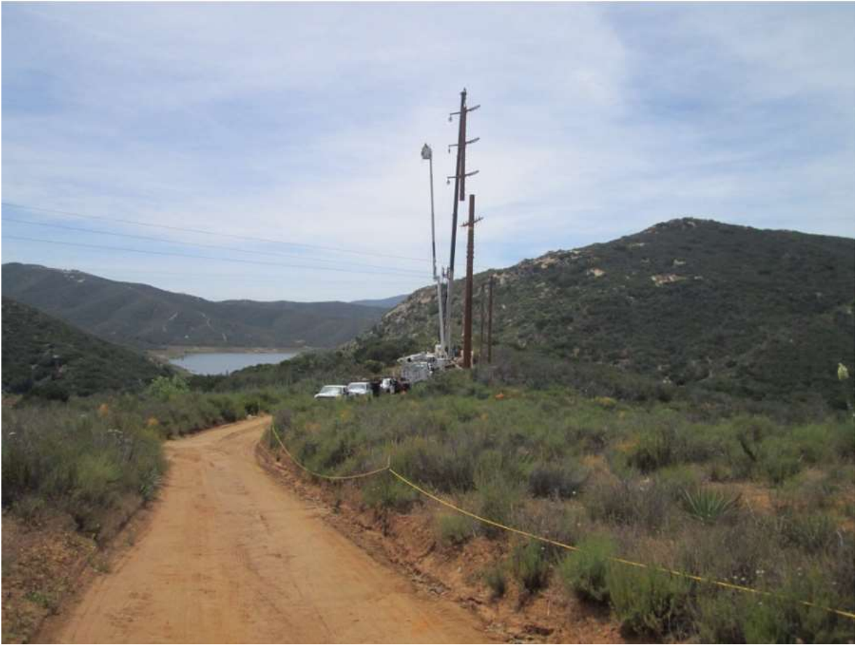
Photo 6: Construction crews were observed setting a steel replacement pole at Pole Z272855 (TL 625B). Environmentally Sensitive Areas were observed roped off for avoidance in accordance with MM CUL-1.
