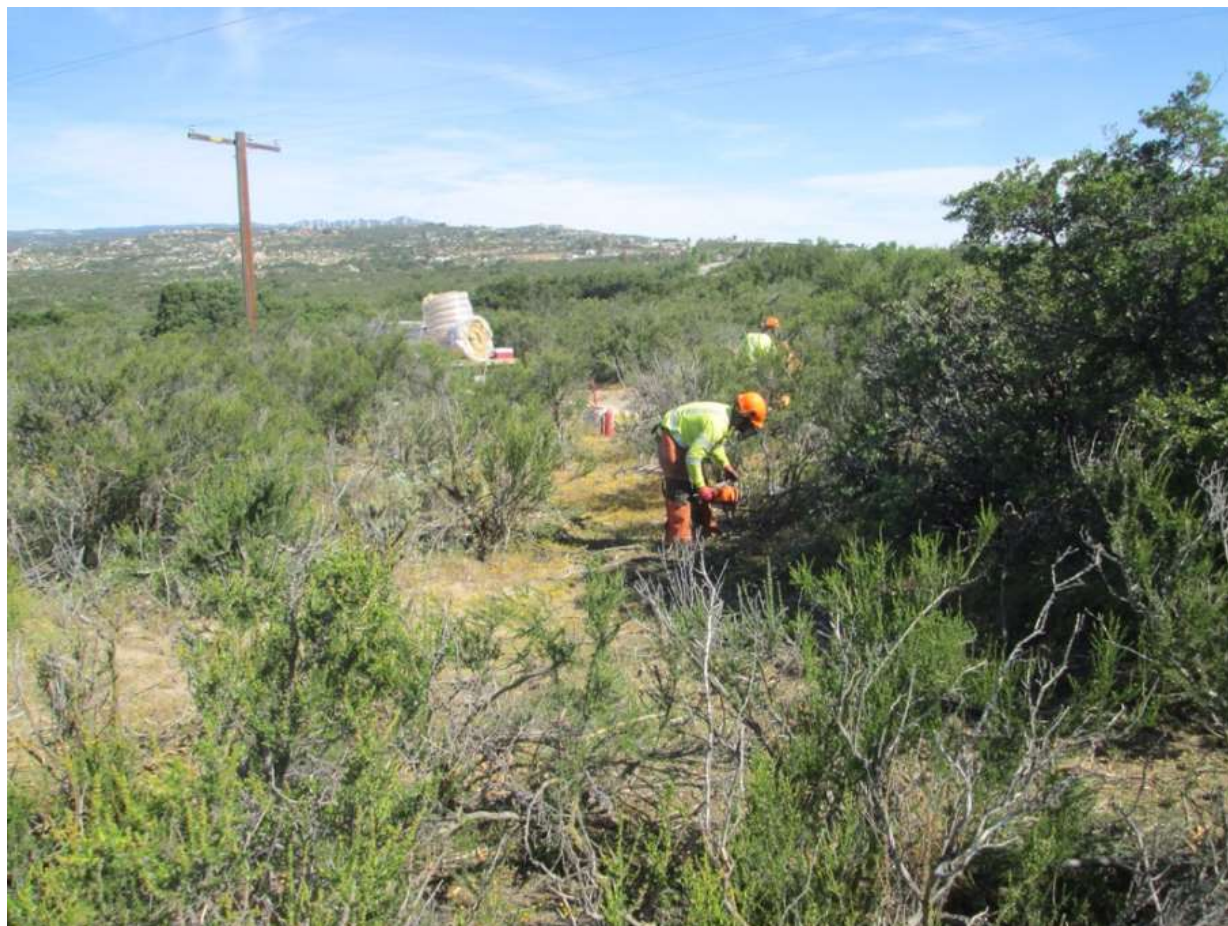
Photo 3: Crews were observed brush clearing at the P46410 Stringing Site (TL 6931). Agave species within the site were flagged and avoided during brush clearing in order to ensure salvage was completed in accordance with the Habitat Restoration Plan (MM BIO-4) and the Special Status Plant Species Salvage and Relocation Plan (MM BIO-15).
