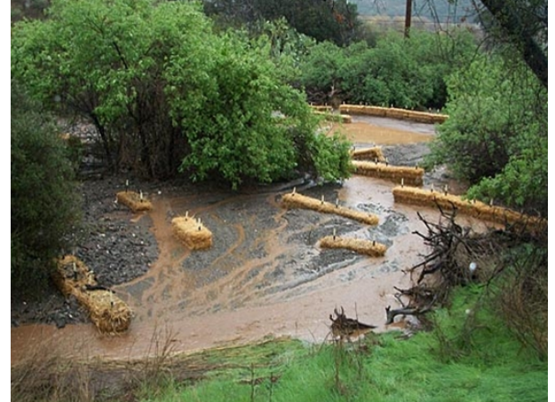
Example of rice hay bales effectively reducing runoff velocity and settling out debris and sediment.
