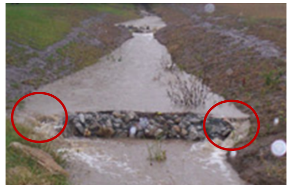
Example of eddies causing erosion around the rock berm.
