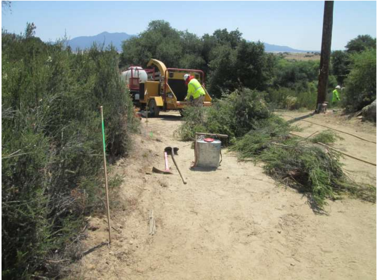
Photo 4: Crews were observed installing SWPPP BMPs (MM HYD-1) and clearing vegetation along TL682 (Location Z118178, above). During vegetation clearing, crews brought required fire suppression equipment in accordance with the CFPPP (MM FF-1) and APM HAZ-01.
