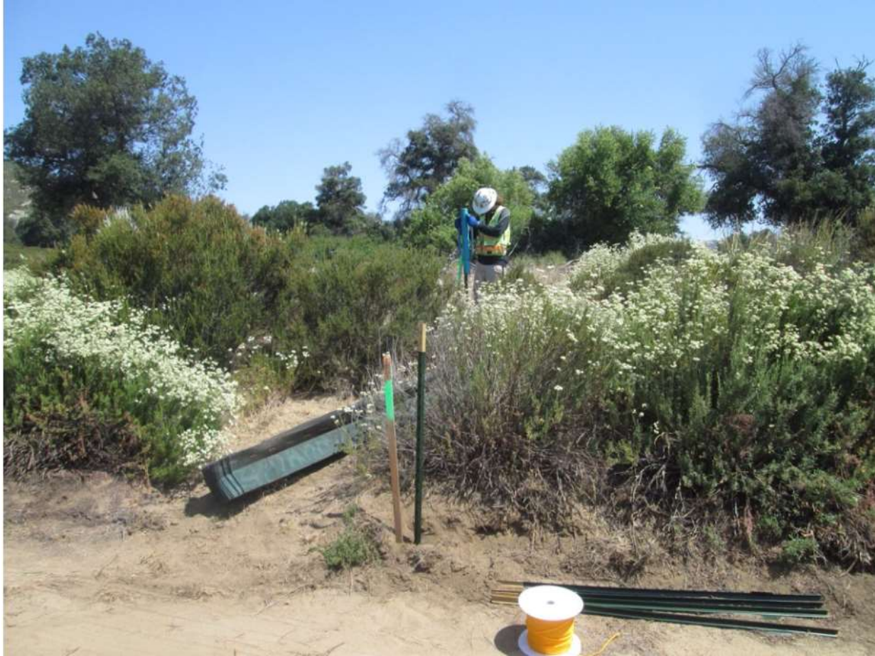
Photo 3: Along TL 682, an archeological monitor was observed installing ESA signage and fencing/rope in accordance with the HPMP (MM CUL-1).
