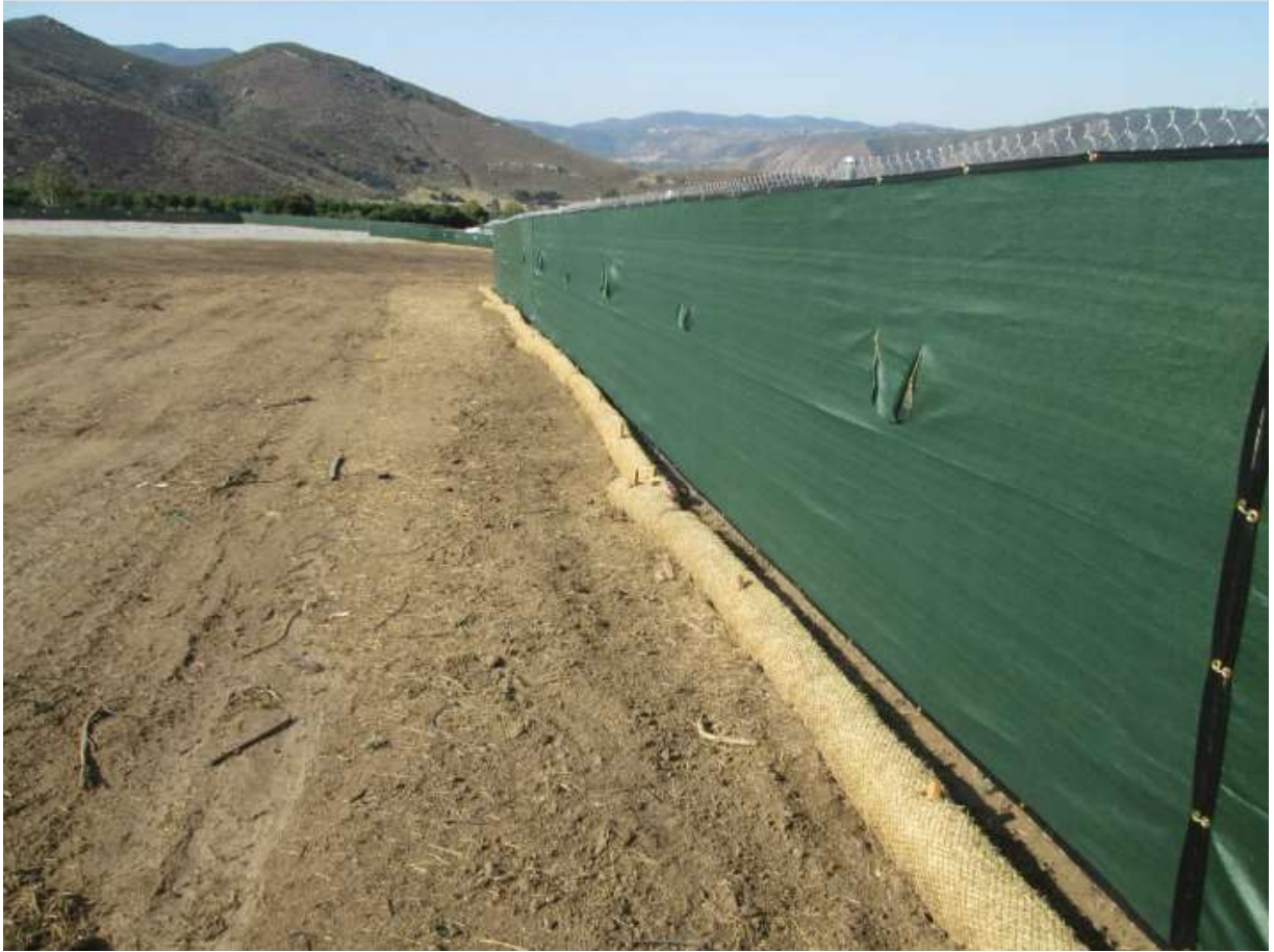
Photo 5: SWPPP BMPs (MM HYD-1) such as fiber rolls and rumble plates were observed at the entrance of the Nursery Staging and Fly Yard (TL 682). Opaque screening material was also observed installed along the yard's perimeter fence in accordance with APM VIS-02.
