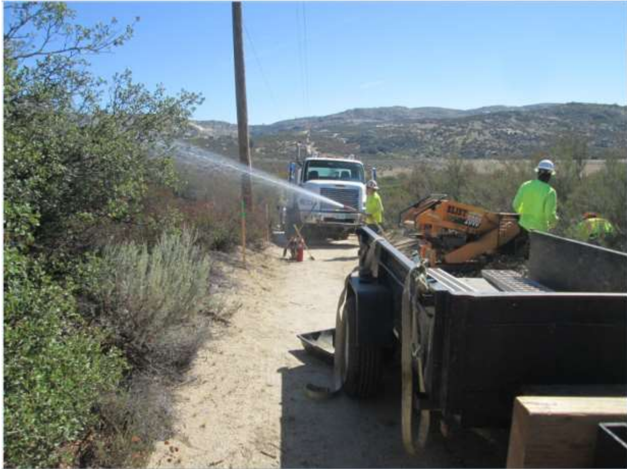
Photo 2: Prior to vegetation clearing, crews were observed watering adjacent areas. Vehicles were observed carrying required fire equipment (5-gallon backpack pump, shovel, Pulaski, and fire extinguisher) and fire equipment was observed staged adjacent to the immediate work areas in accordance with the CFPPP and APM HAZ-04.
