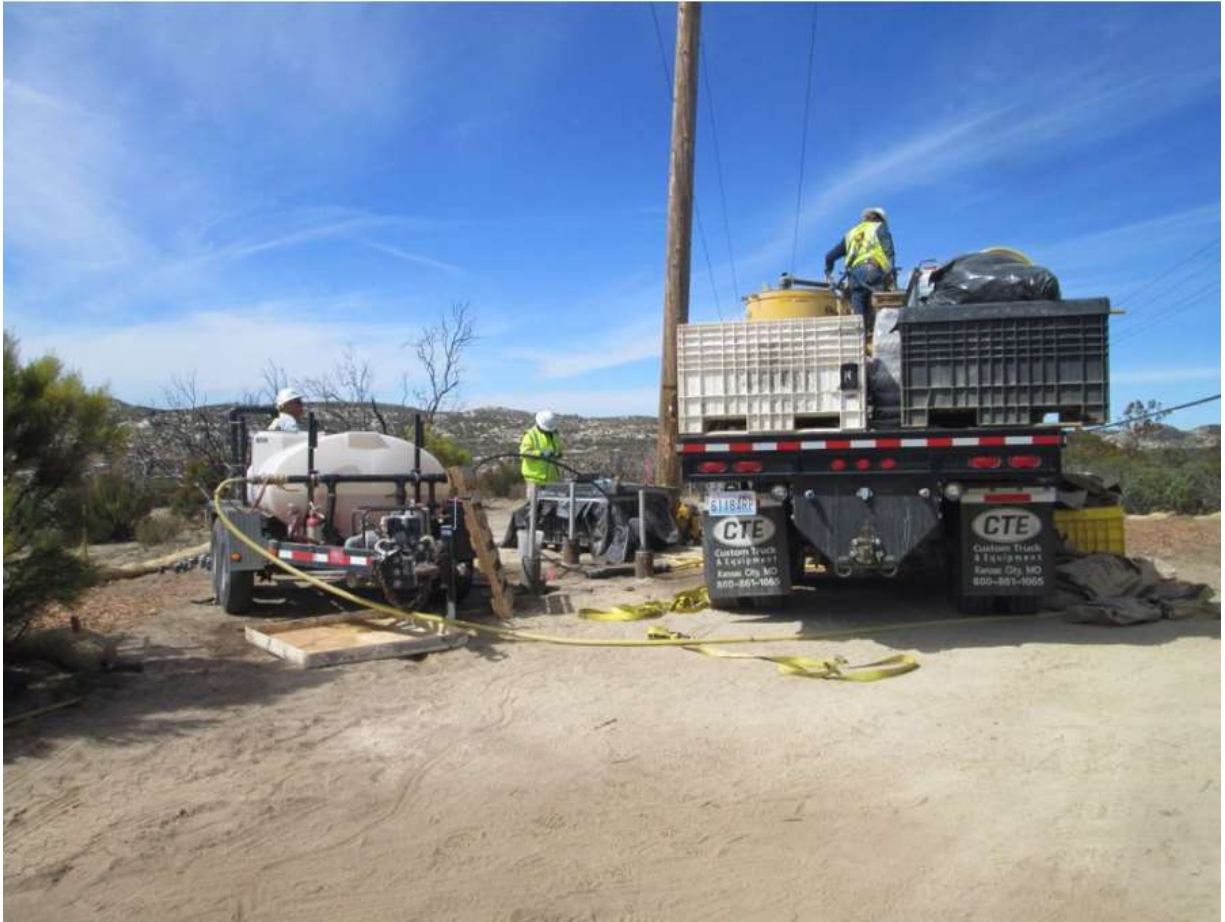
Photo 4: Crews were observed grouting micropile foundations subsequent to foundation drilling. Work was observed being conducted within staked work limits and spill kits were observed present in accordance with MM PHS-2.
