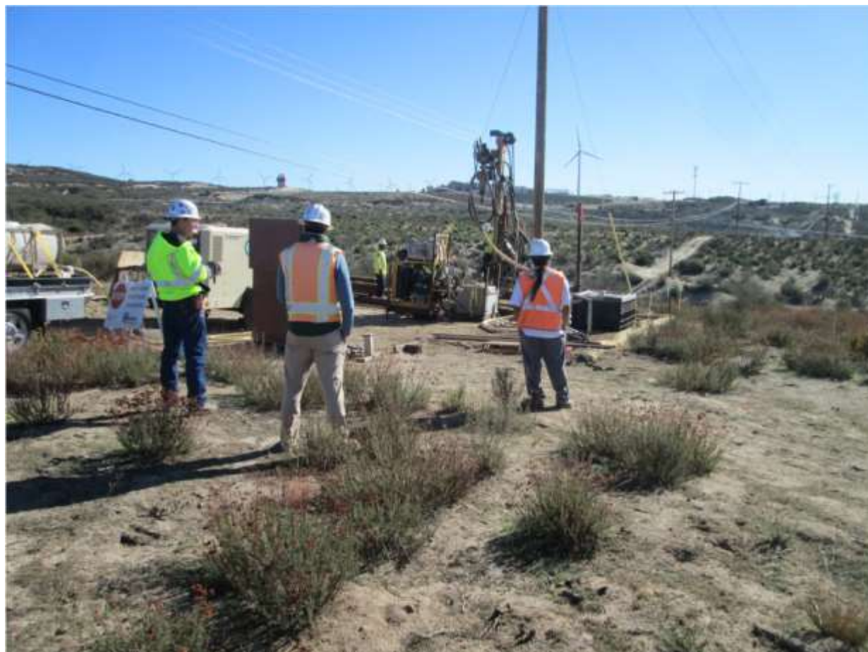
Photo 3: During applicable micropile activities, biological, cultural, and Native American Monitors were approved present in accordance with MM BIO-3 and APM CUL-4 and MM CUL-3. Staking of approved work areas was observed in accordance with MM BIO-22.
