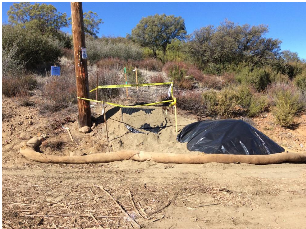
Photo 2: Following drilling at pole P176946 (C 442), the pole hole was securely covered in accordance with MM-BIO-23 and spoils were contained within a tarp in accordance with the Erosion Control Plan.
