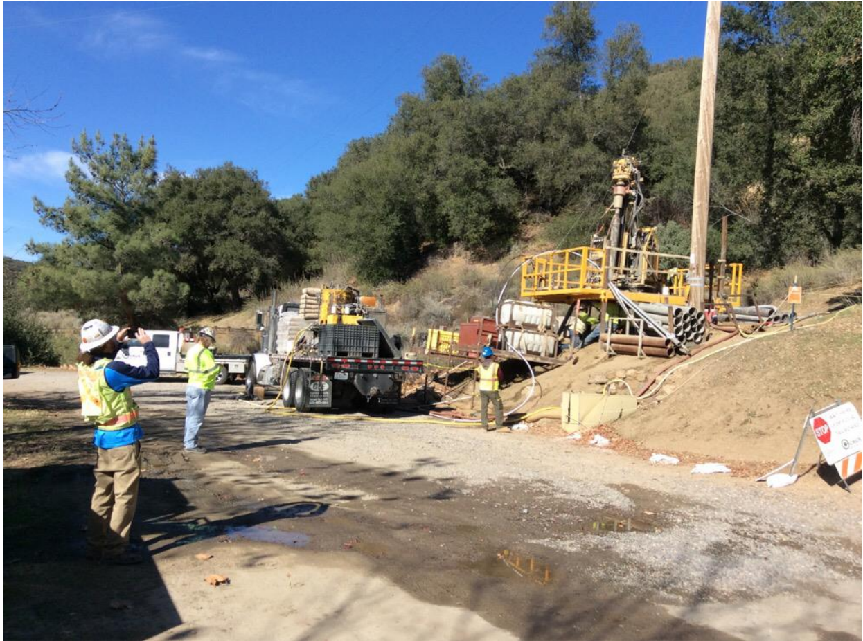
Photo 5: Biological and archeological monitors were observed monitoring the grouting activity at pole Z118106 (TL 682).
