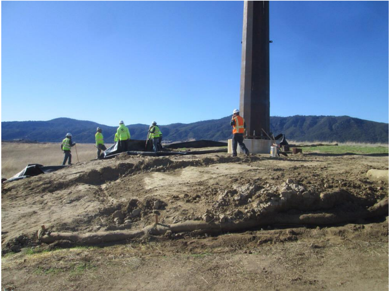
Photo 4: An Icon crew observed deconstructing and removing SKR exclusion barrier at Z118190 (TL 682).
