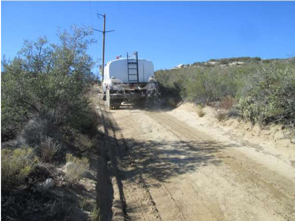
Photo 4: Water trucks were observed applying water to work areas and access roads along TL 629E to minimize fugitive dust in accordance with APM AIR-02.
