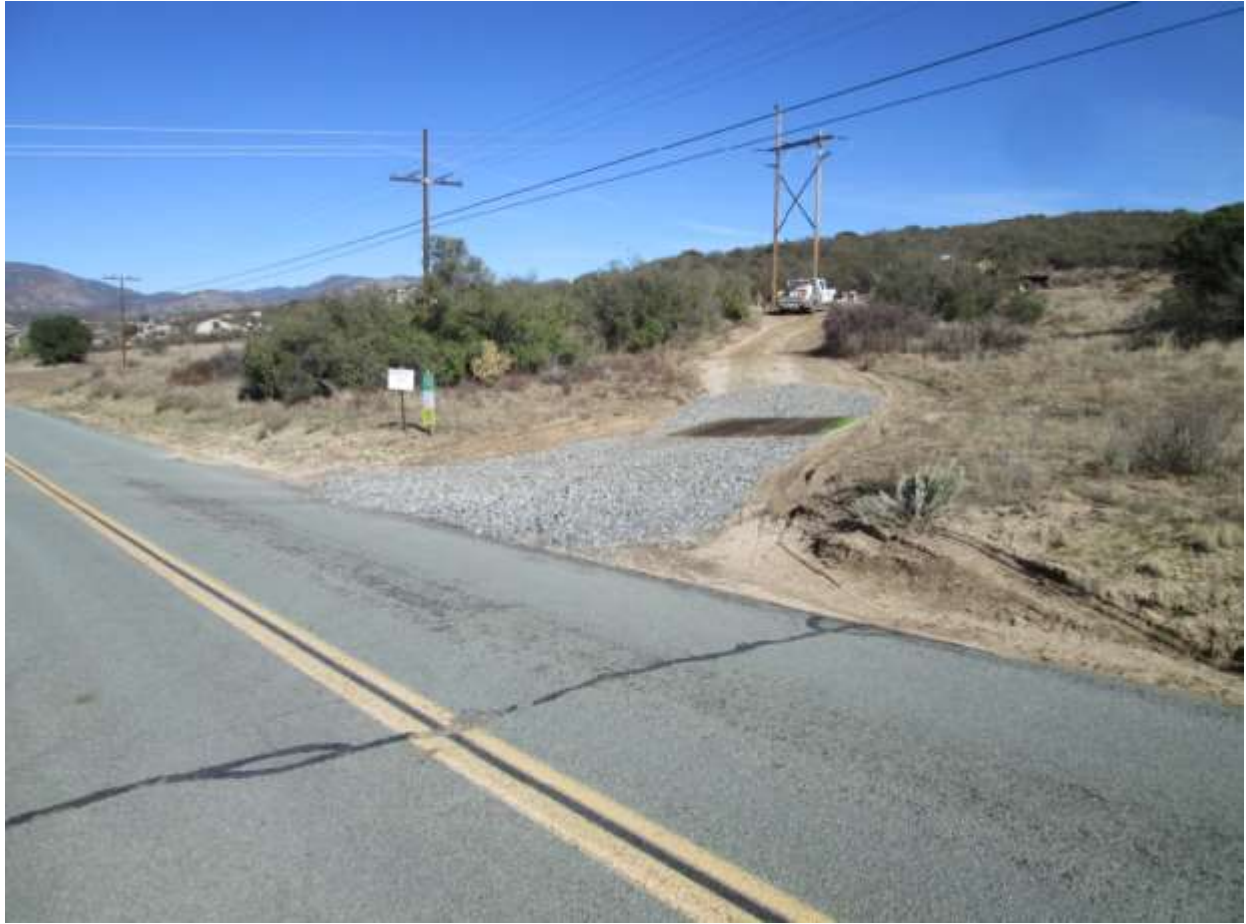
Photo 5: A rock apron and rumble plate were observed at an entrance to the TL 629E ROW in order to minimize sediment track out onto paved roadways in accordance with the SWPPP (APM HYD-05, MM BIO-7, and MM HYD-1).
