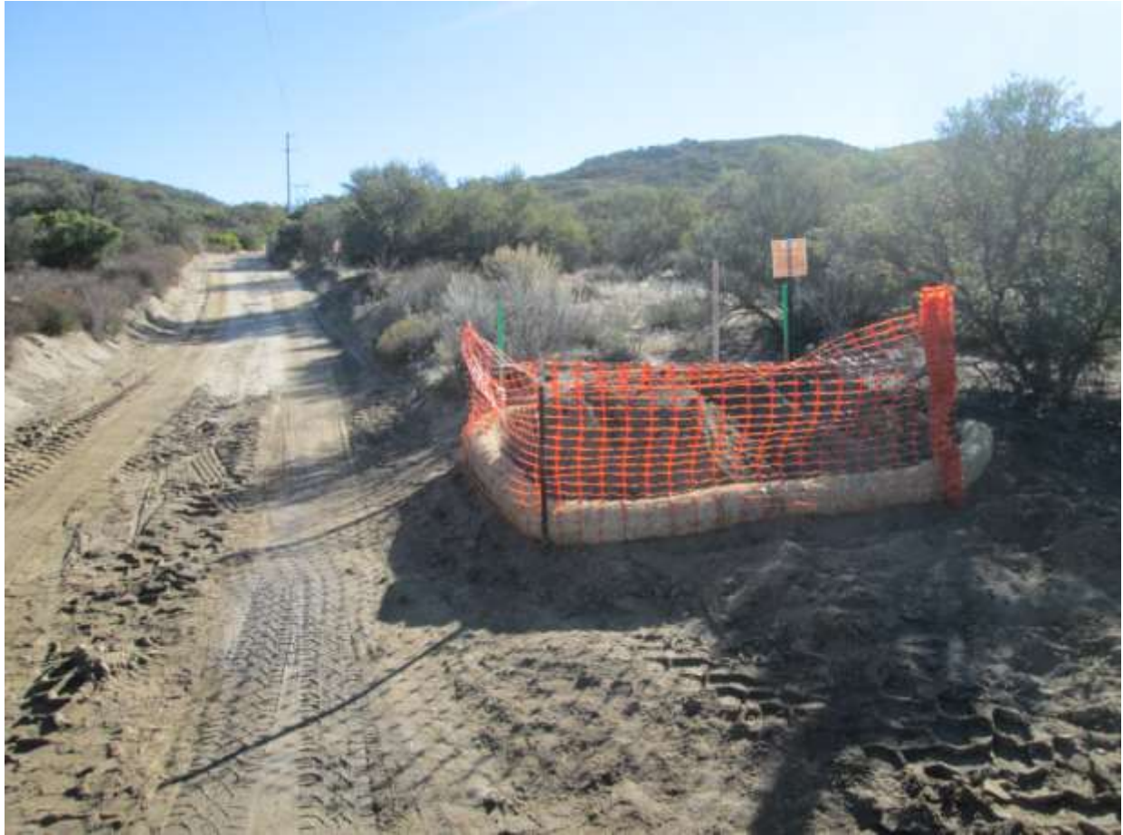
Photo 3: Topsoil was observed salvaged along TL 629E (adjacent to Pole Z44176, above) in accordance with MM BIO-4 and the Habitat Restoration Plan. Stockpiles were surrounded by fiber rolls in accordance with the Erosion Control Plan and project SWPPP.
