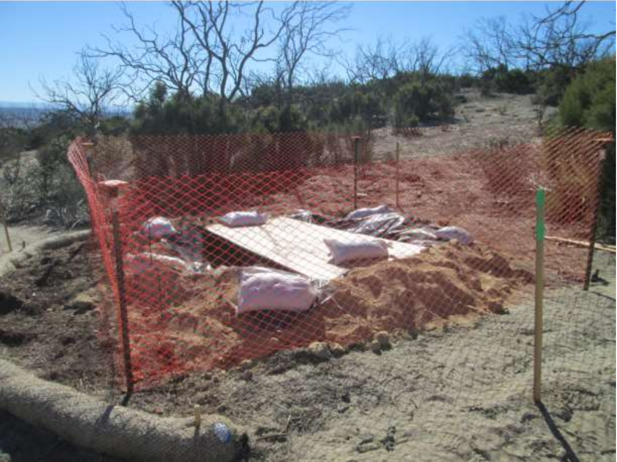
Photo 2: Upon completion of auguring along TL 629E, open holes were observed covered to prevent wildlife entrapment in accordance with MM BIO-23.
