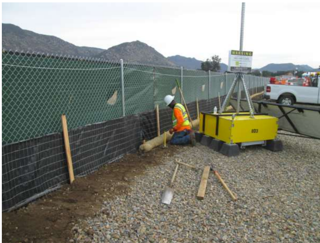
Photo 6: Construction crews were observed installing arroyo toad exclusion fence along the inside perimeter fence at the Anderson Staging Yard in accordance with the Streambed Alteration Agreement.
