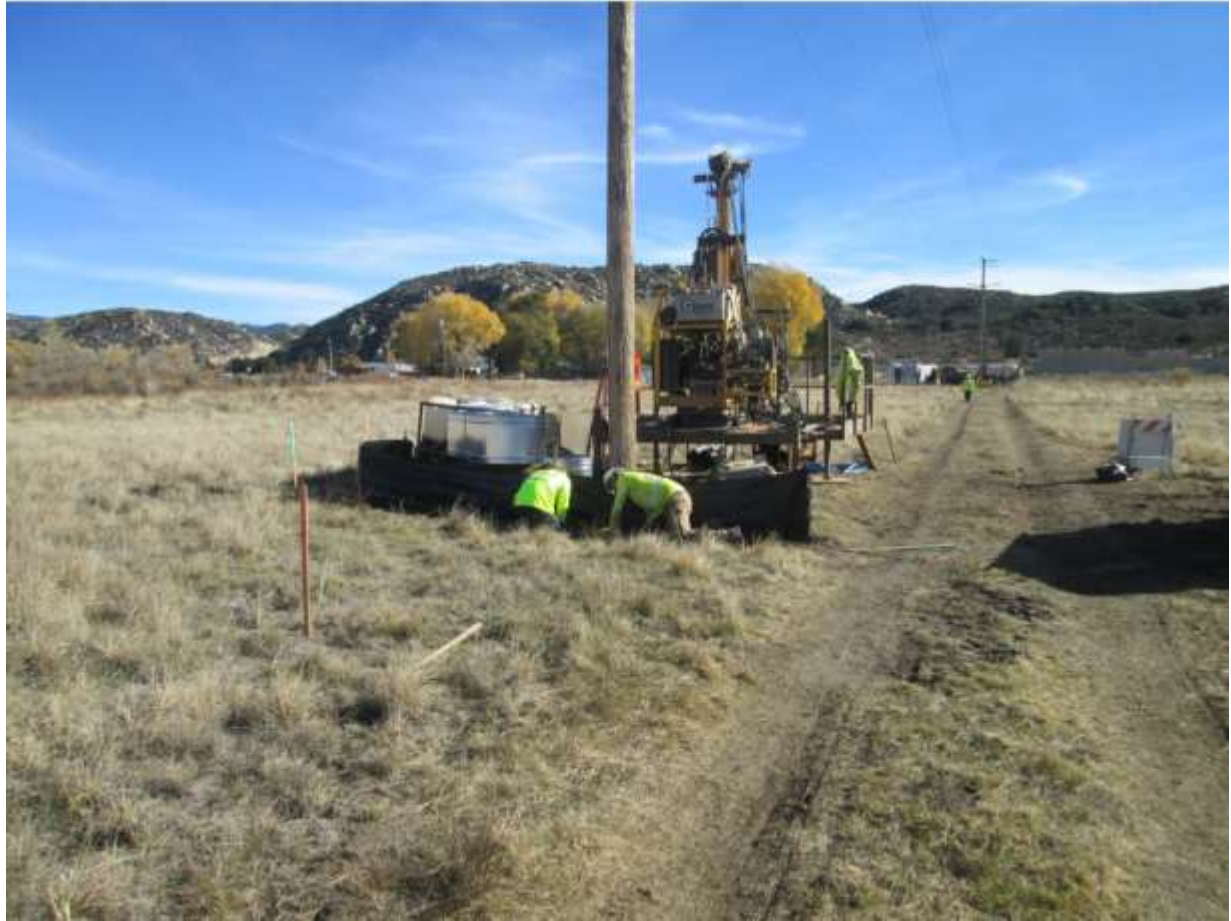
Photo 3: Crews were observed preparing for microile drilling activities along TL 629E (Pole Z44158, above) and installing silt fencing in accordance with the SWPPP.
