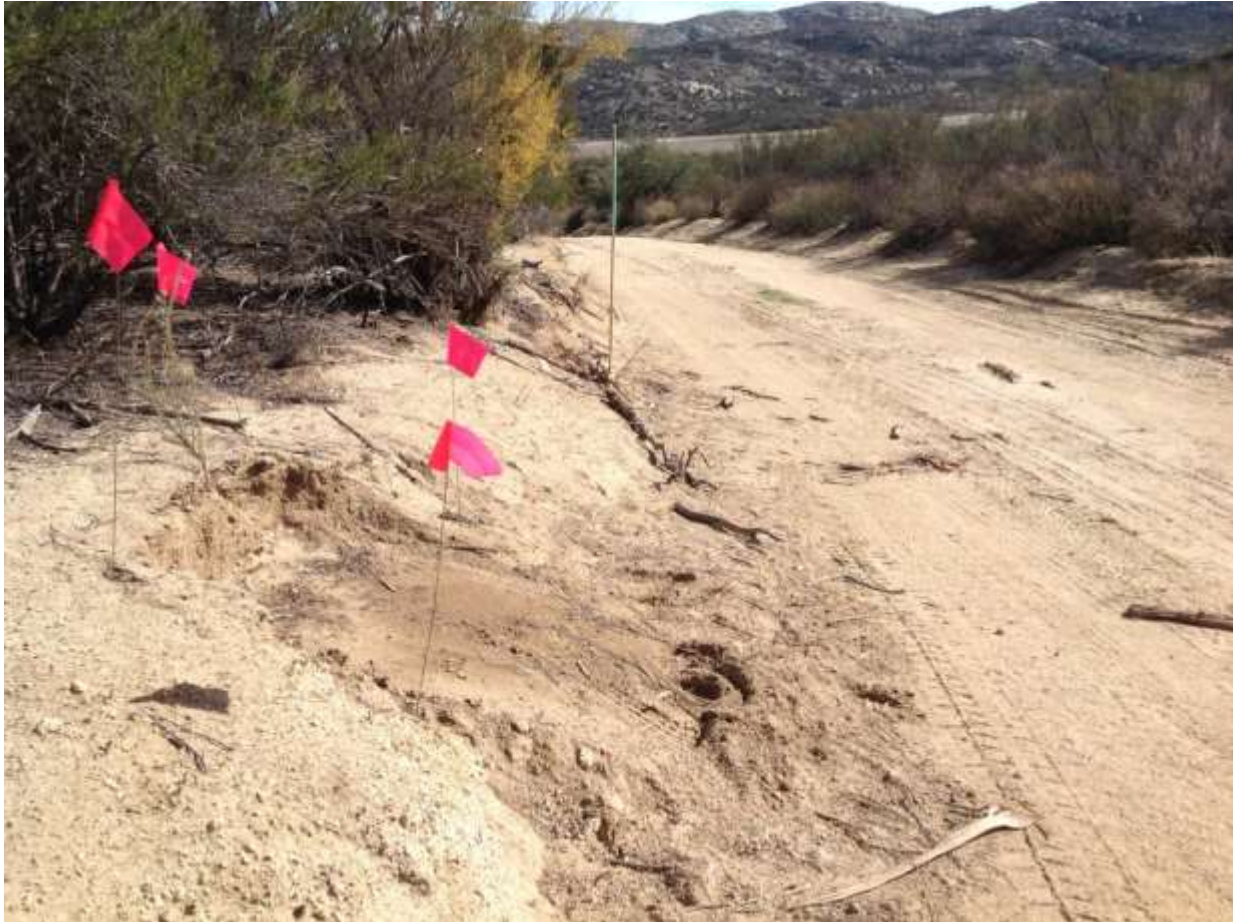
Photo 6: Following the Minor Deviation issued by CPUC on December 12, 2016, monitors flagged areas where crane foot pads were staged in order to ensure compensation and restoration was tracked in accordance with APM BIO-3, and MM BIO-4 and 5 (above, adjacent to Pole Z44199).
