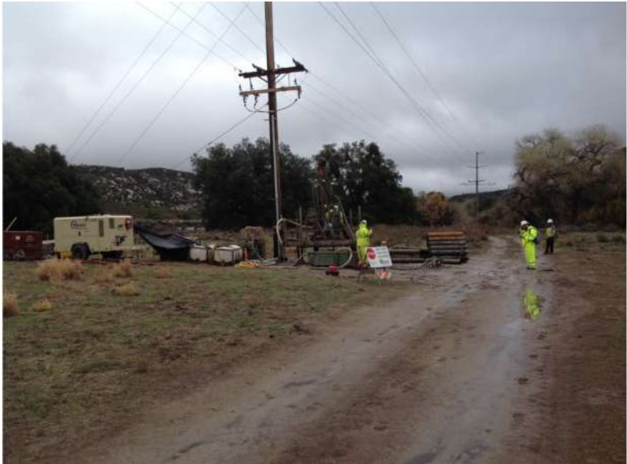
Photo 5: Sediment rotary tanks were observed installed at work sites to assist with drilling and to alleviate pooling groundwater within workspaces along TL 629E (Pole location Z40582, above).
