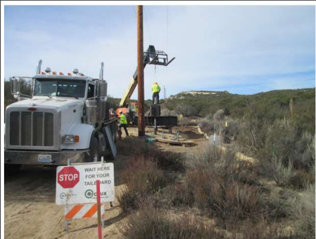
Photo 1: Crews were observed strength testing micropile foundations along TL 629E (Pole Z44169, above). Crews were observed staying within the delineated work limits (MM BIO-1) and ESAs were observed marked for avoidance in Quino Checkerspot Butterfly habitat (MM BIO-21).
