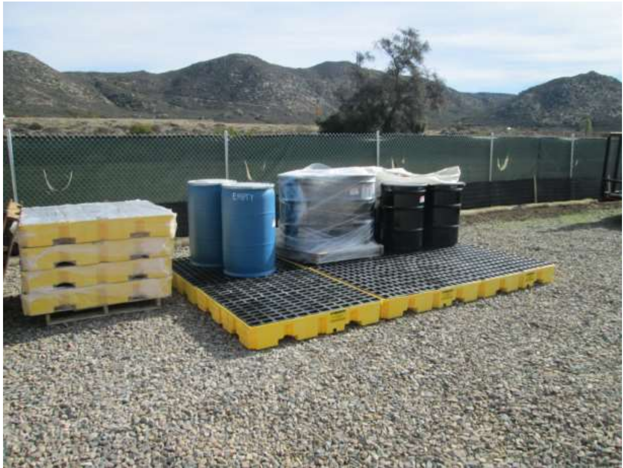
Photo 2: Hazardous materials were labeled and stored at staging yards in accordance with MM PHS-2.
