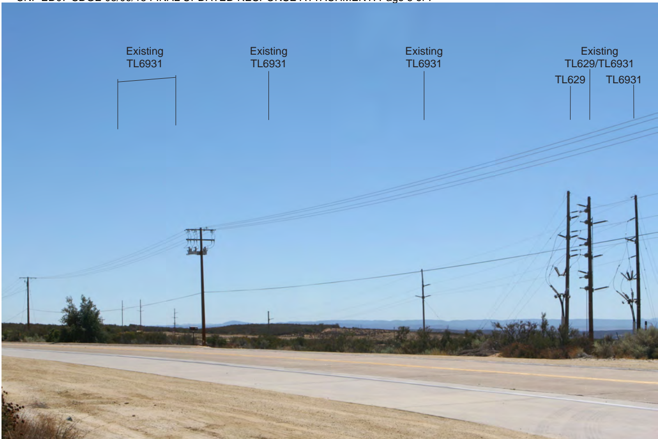
Existing view from Crestwood Substation looking southeast (KOP 16)
