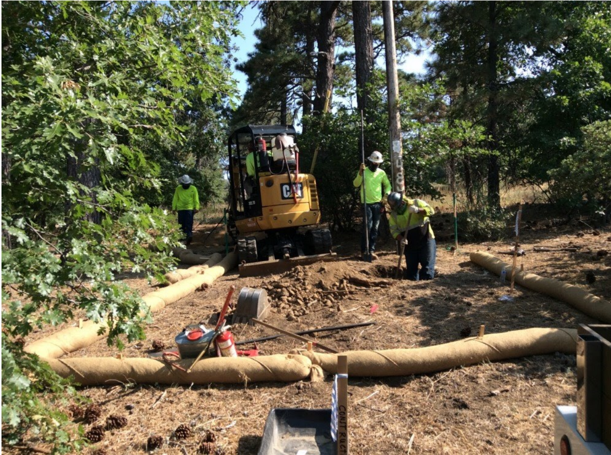
Photo 6: A crew was observed digging a direct bury pole hole and digging an anchor excavation at Pole P40245 (C 440). Site-specific erosion control BMPs were observed in good condition in accordance with the ECP, SWPPP (MM HYD-1 and MM BIO-7), and APM HYD-09.
