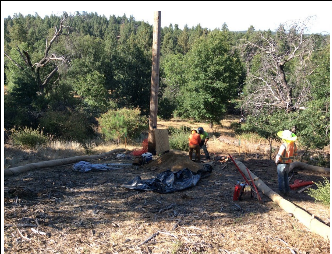
Photo 3: In accordance with APM CUL-08, a Paleontological Monitor was observed monitoring excavations at locations with underlying Potential Fossil Yield Classification Class 3 geologic deposits where new poles were unable to be installed in the same location as the existing poles along C 440.
