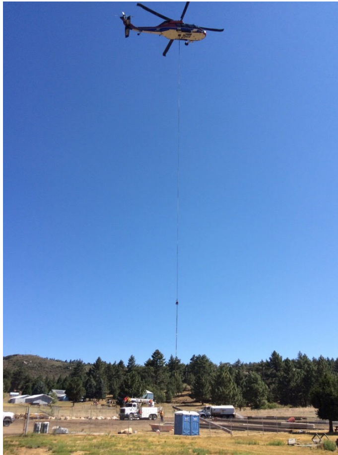
Photo 1: A water tender was observed applying water to the surface at Morris Ranch Staging Yard (C 440) before and during helicopter activities to minimize dust emissions from rotor wash in accordance with APM AIR-02 and the Aviation Safety Plan (MM PHS-5).
