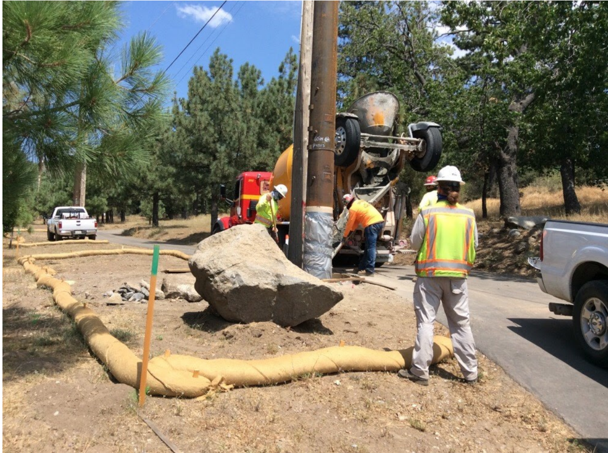
Photo 2: A crew was observed pouring concrete at Pole P45113 (C 440). A Biological Monitor was observed monitoring construction activities along the alignment to ensure compliance with mitigation measures, applicant proposed measures, and permit conditions in accordance with MM BIO-22.
