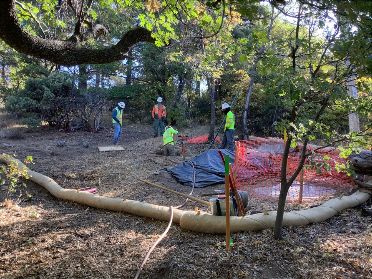
Photo 6: During anchor excavation at Pole P40392 (C 440), site-specific erosion control BMPs were observed in good condition in accordance with the ECP and SWPPP (MM HYD-1) and APM HYD-09.
