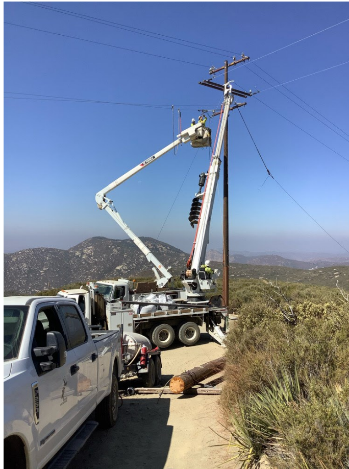
Photo 4: During overhead line work associated with wire stringing at Pole P258564 (C 79B), a Designated Fire Patrol was present and equipped with at least 150 gallons of water with pump and hose in accordance with the CFPPP Fire Prevention Matrix for conductor work with de-energized lines on USFS land with a PAL D.
