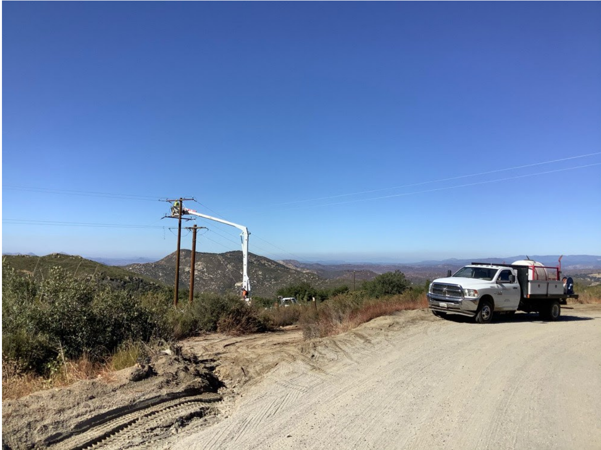
Photo 3: A Designated Fire Patrol was present during overhead work at Pole P258558 (C 79B) in accordance with the CFPPP for conductor work with energized lines off NFS land with a Normal FPI.
