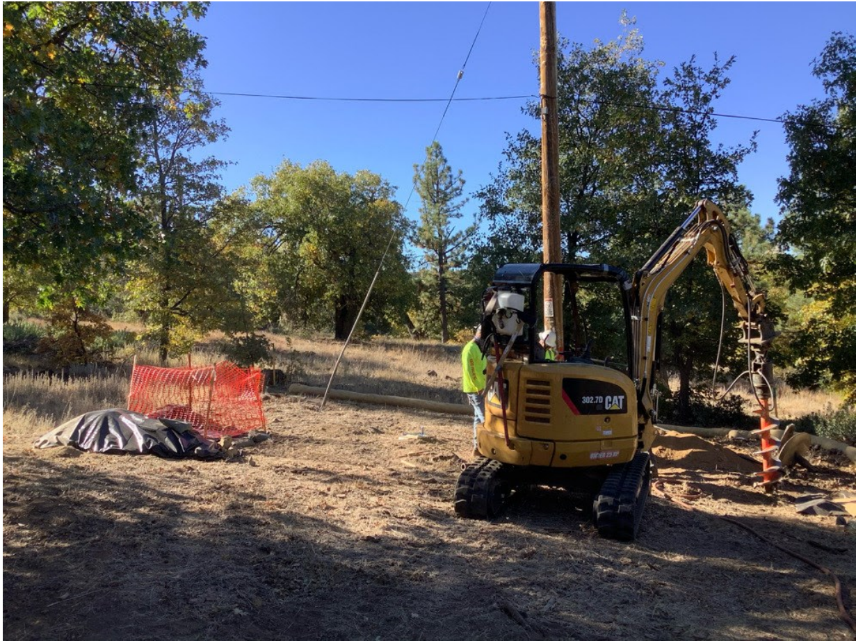
Photo 5: A crew was observed drilling a pole hole at Pole P40470 (C 440). An anchor excavation at the site was observed to be covered to prevent wildlife entrapment in accordance with MM BIO-23, and the associated spoils stockpile was observed to be covered in accordance with the ECP, SWPPP, and APM HYD-09.
