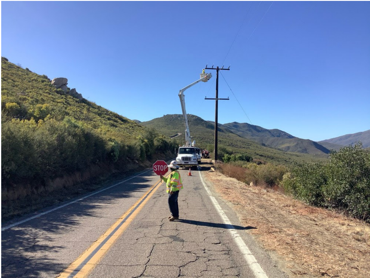
Photo 6: Cones, signage, and flagpersons were used to direct one-way traffic on Boulder Creek Road during construction activities at Pole P258511 (C 79B) in accordance with APM TRANS-02.
