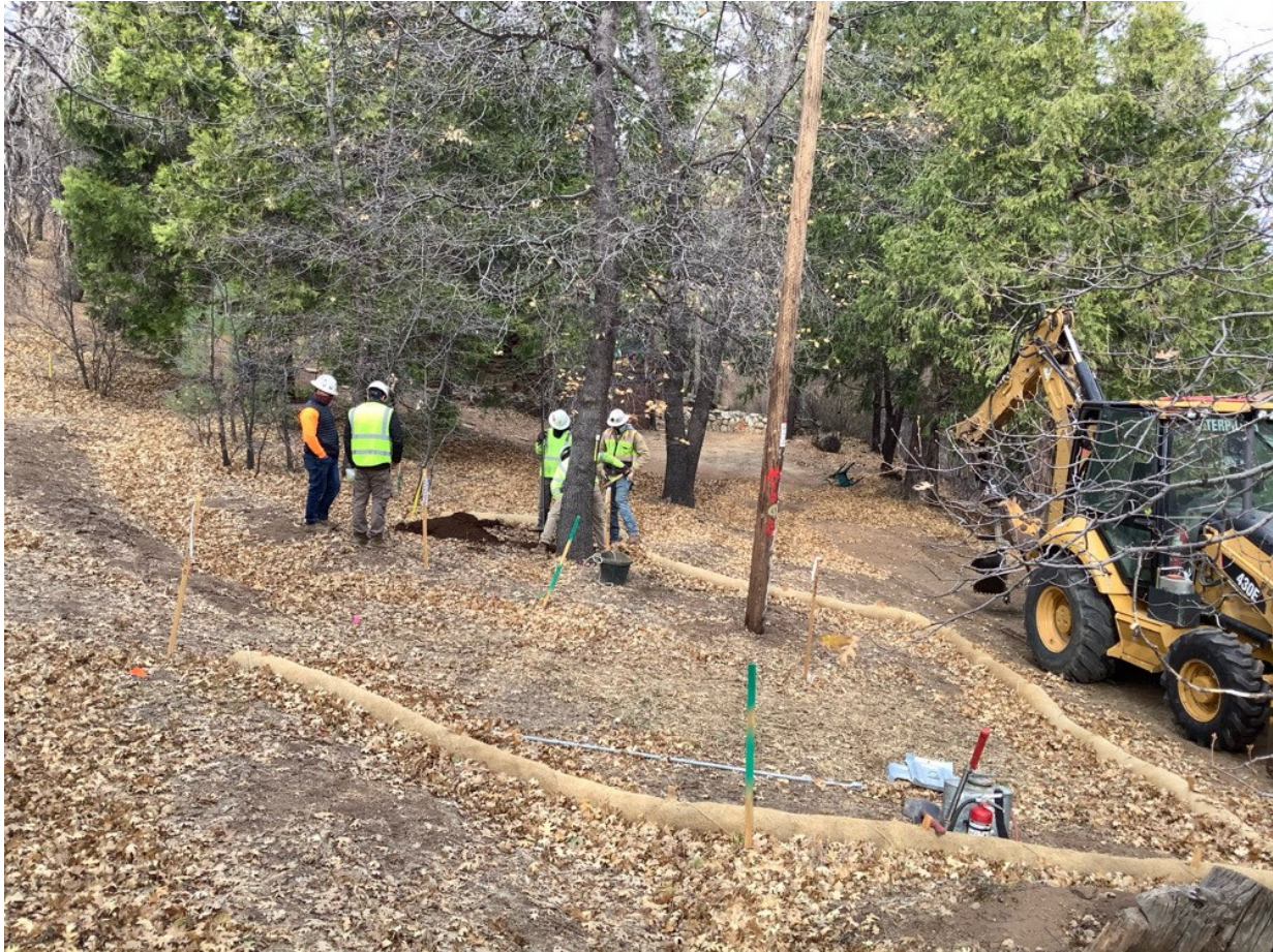
Photo 3: Archaeological and Cultural Monitors were observed monitoring anchor excavation along C 440 in accordance with the HPMP, MM CUL-1, MM CUL-3, and APM CUL-04.
