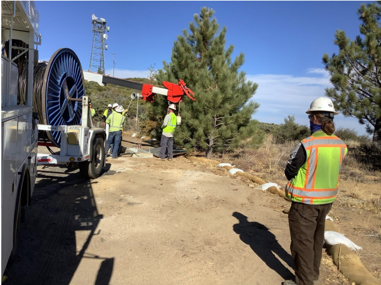
Photo 2: A Biological Monitor was observed monitoring underground cable pulling (C 440) to ensure compliance with mitigation measures, applicant proposed measures, and permit conditions in accordance with MM BIO-22.
