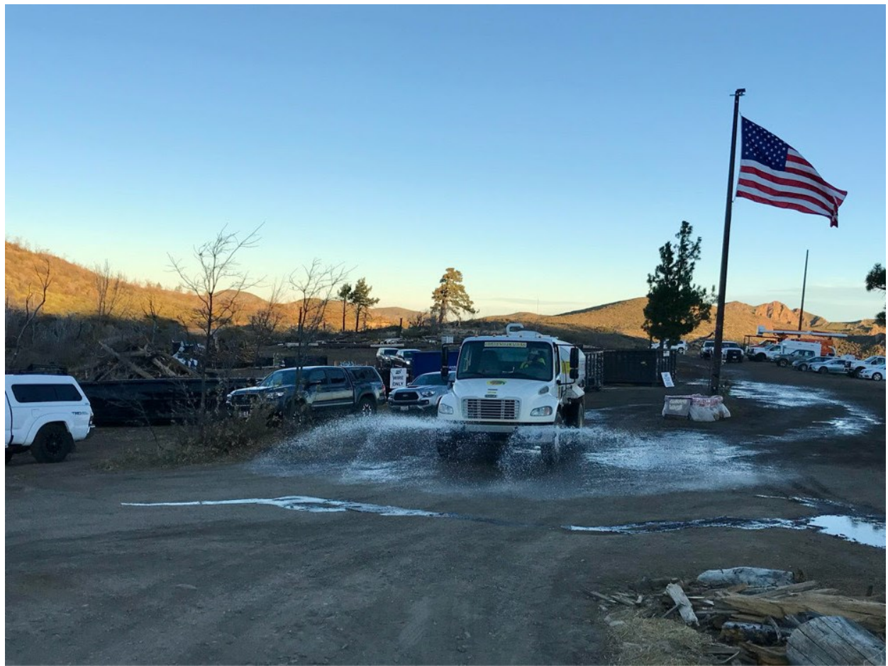
Photo 1: A water tender was observed applying water to the surface at Shrine Camp Staging Yard (C 440) in the morning to reduce dust emissions during crew egress in accordance with APM AIR-02.
