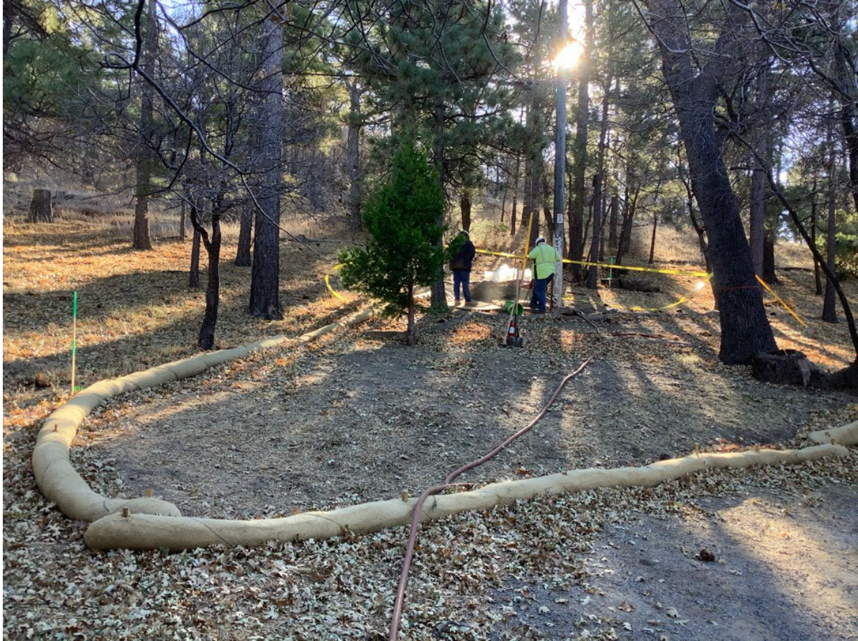
Photo 5: During pole hole excavation at Pole P40351 (C 440), erosion control BMPs were observed in good condition in accordance with APM HYD-09, the ECP, and the SWPPP (MM HYD-1 and MM BIO-7).
