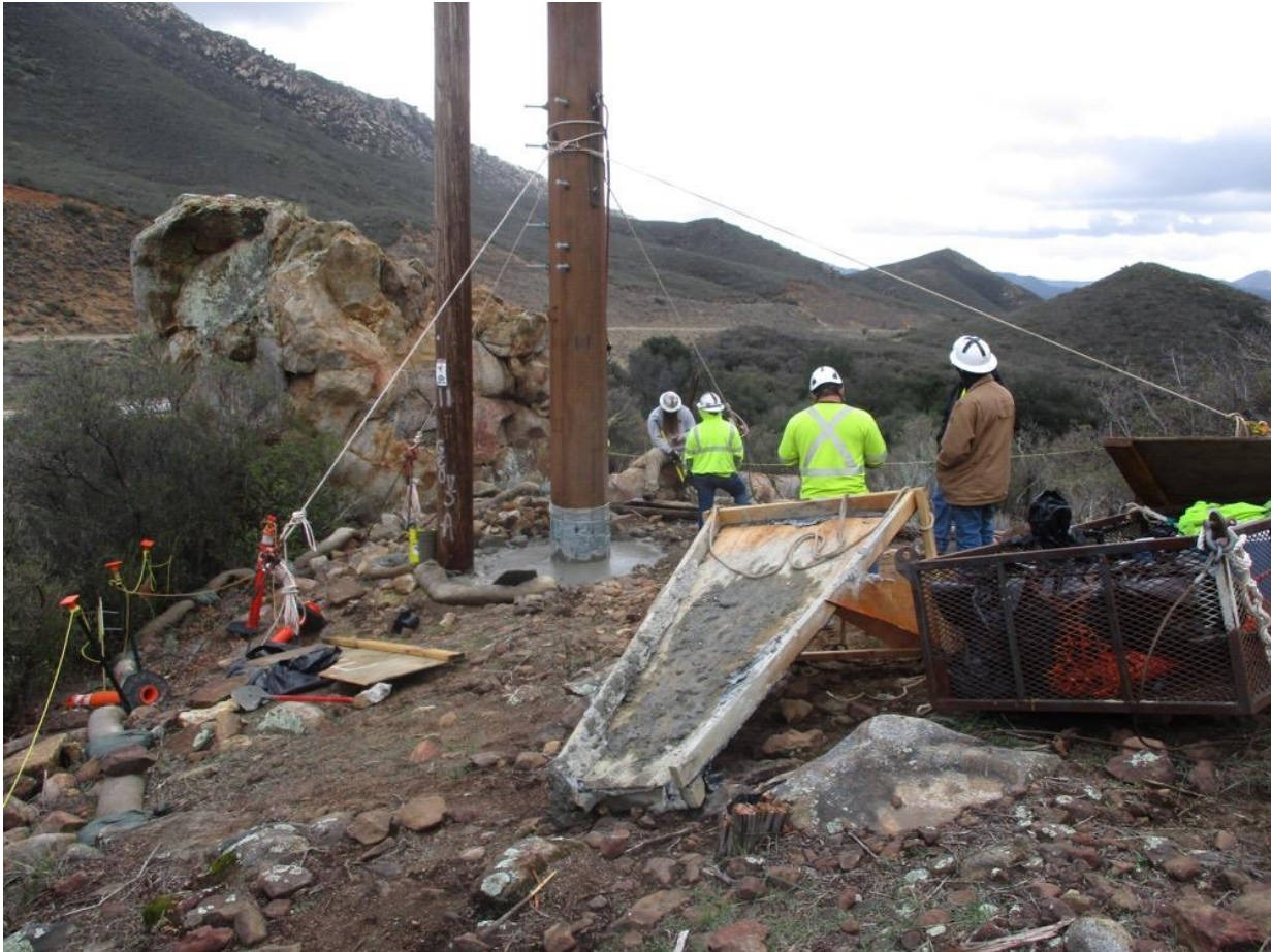
Photo 3: BMPs were implemented during direct bury foundation pouring at Z40425 (TL 629C) including fiber rolls and concrete waste containment to prevent excess concrete and waste from being discharged onto the ground in accordance with APM HYD-01.
