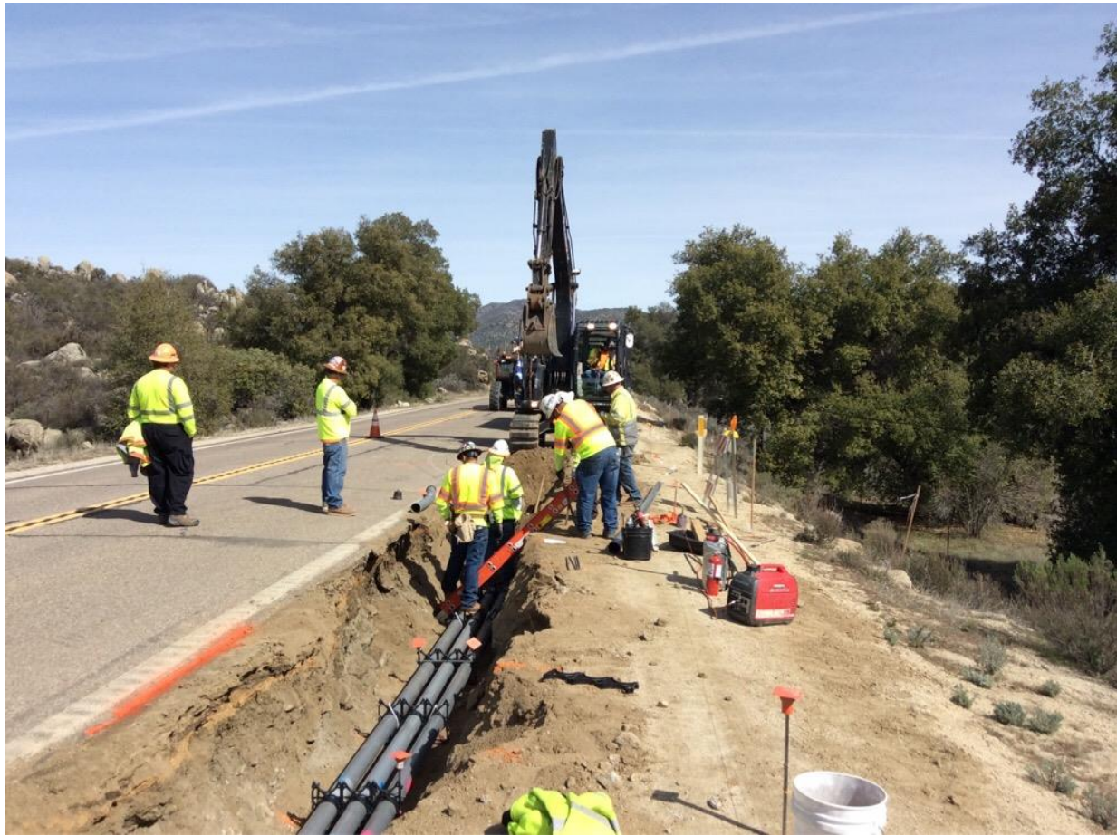
Photo 5: Construction crews were observed trenching and installing conduit along Buckman Springs Road (C 449).
