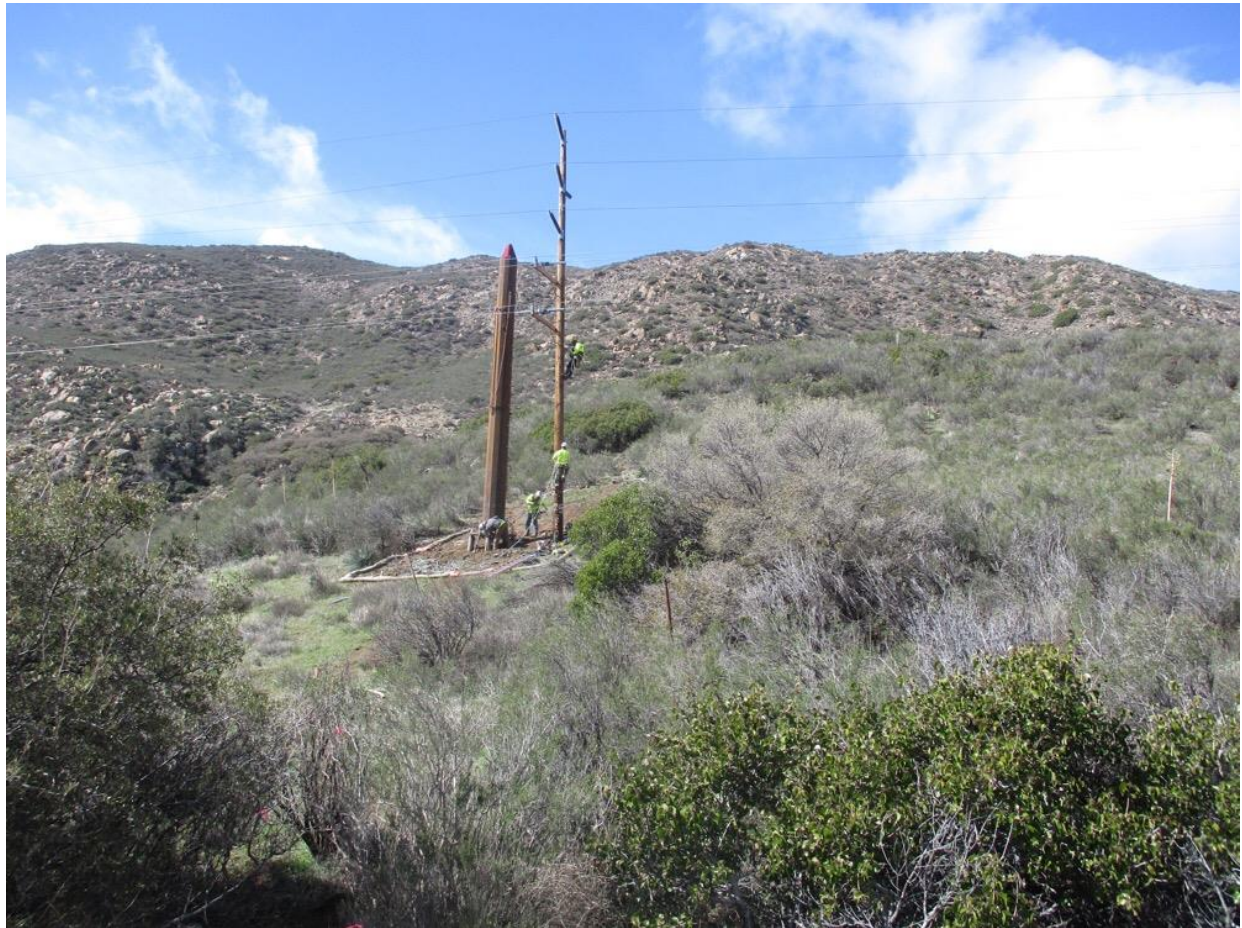
Photo 2: A construction crew was observed installing a pole base recently delivered via helicopter external load and preparing to receive the pole top at Z40511 (TL 629C).
