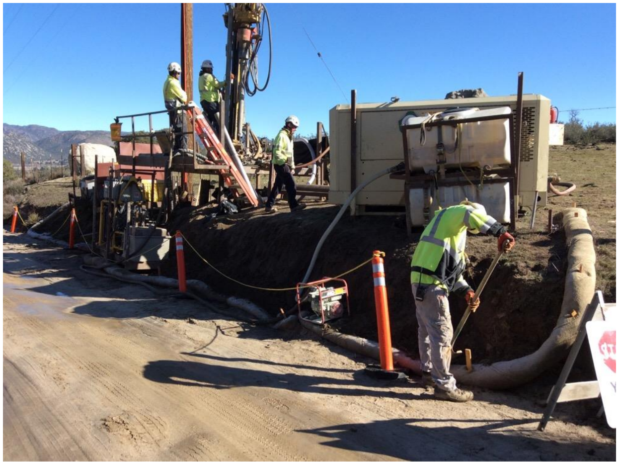
Photo 1: A construction crew was observed conducting sediment and erosion control BMP maintenance at Pole Z40990 (TL 6958) during micropile foundation drilling in accordance with the Erosion Control Plan and SWPPP.
