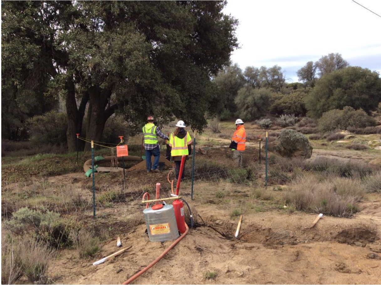
Photo 2: Project personnel were observed avoiding a clearly marked ESA surrounding the anchor at Pole P258862 (C 449) in accordance with the HPMP and APM CUL-03. In addition, Archaeological and Cultural Monitors were present in accordance with APM CUL-04 and MM CUL-1.
