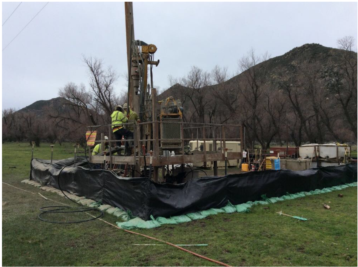
Photo 1: A construction crew was observed setting rebar at Pole Z40980 (TL 6958). The lower portion of the Arroyo toad fencing surrounding the site was observed to stretch outward along the ground and be secured with a continuous line of gravel bags in accordance with the Arroyo Toad Monitoring and Relocation Plan.
