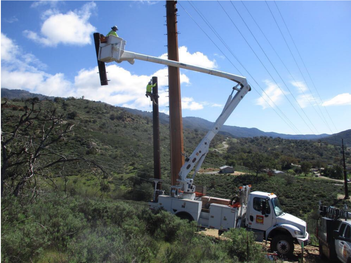
Photo 6: A construction crew observed cutting the old pole at Z118069 (TL 682) and loading pieces onto a truck for off-site hauling. The crew was observed working within the approved work space in accordance with MM BIO-1.
