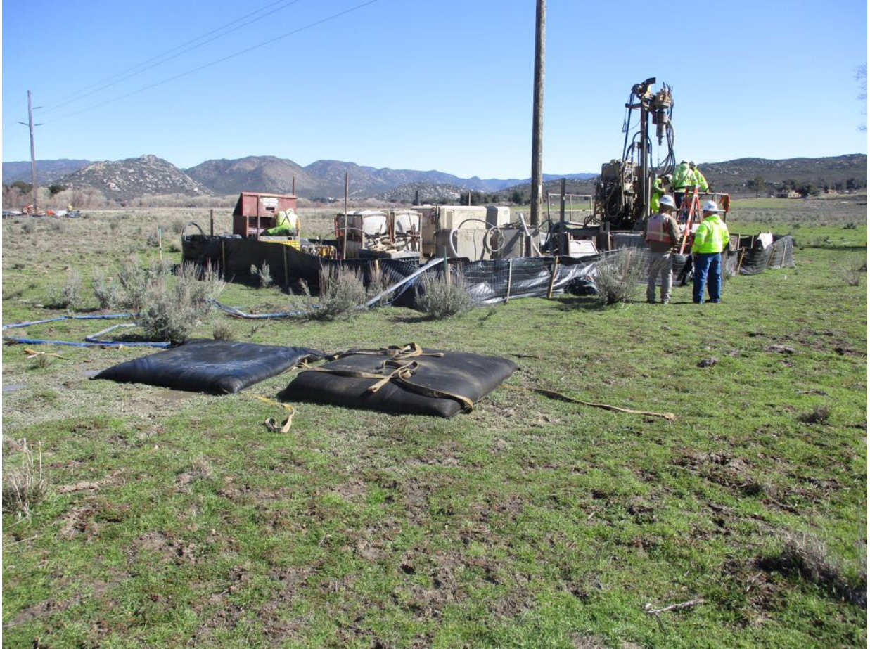
Photo 3: A construction crew observed drilling for a micropile foundation at Pole Z40979 (TL 6958). Ground water encountered while drilling was pumped into tanks and through filter bags before being discharged to land in accordance with APM HYD-08.
