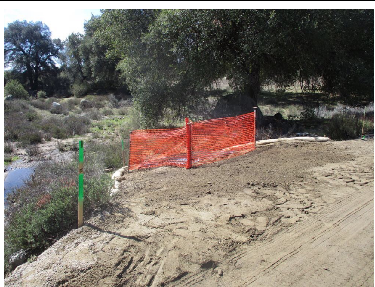
Photo 4: To prevent erosion of dirt spoil (from pole hole drilling) into a nearby jurisdictional drainage adjacent to P258855 (C 449), a construction crew removed the dirt spoil and cleaned-up/raked, and removed sediment buildup on fiber rolls in accordance with the ECP, SWPPP, and SAA. Work limits were clearly delineated in accordance with MM BIO-1.
