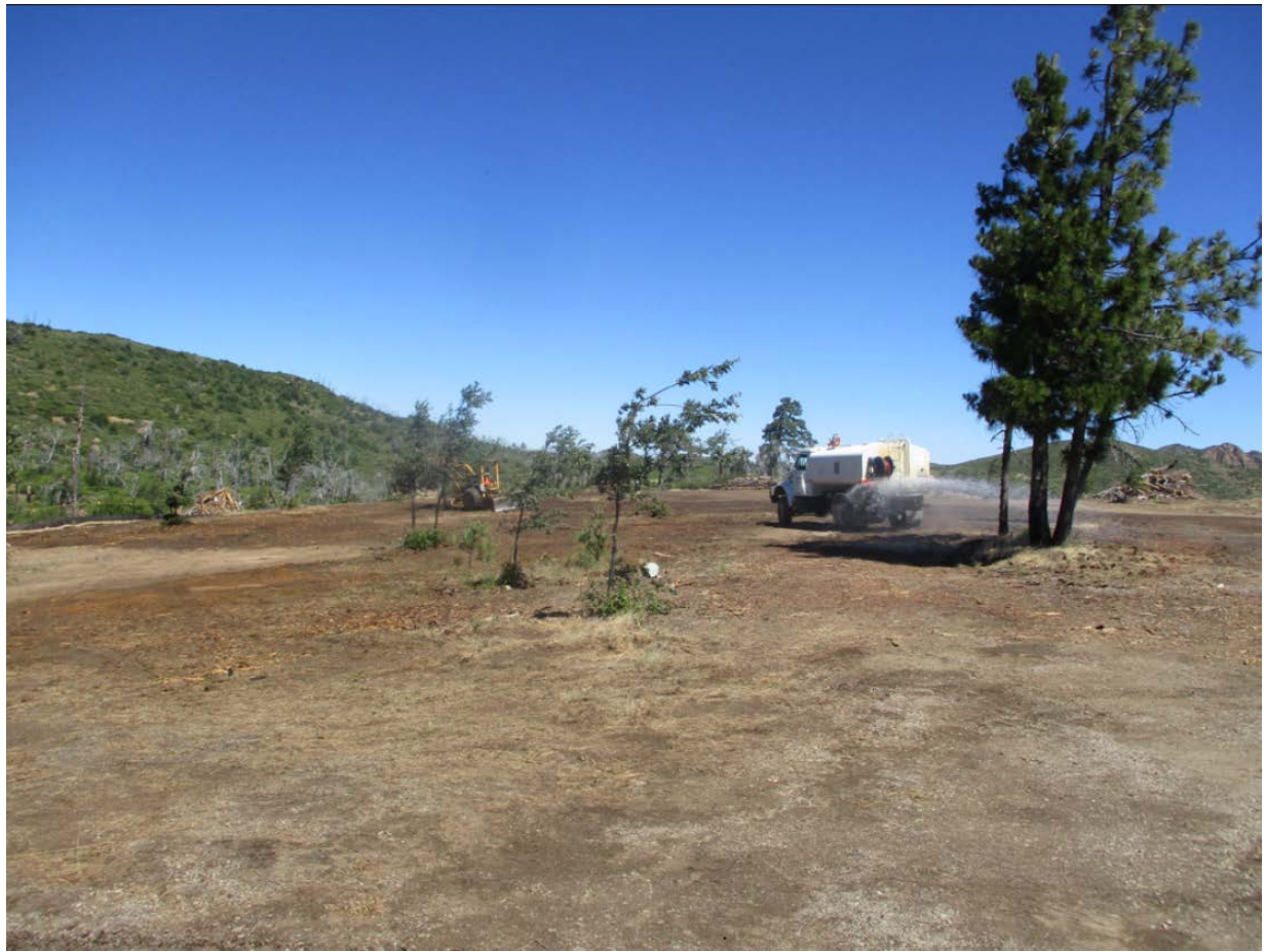
Photo 1: A crew was observed conducting grading work at Shrine Camp Staging Yard. Water was applied to prevent dust emissions in accordance with APM AIR-02 and APM AIR-05.
