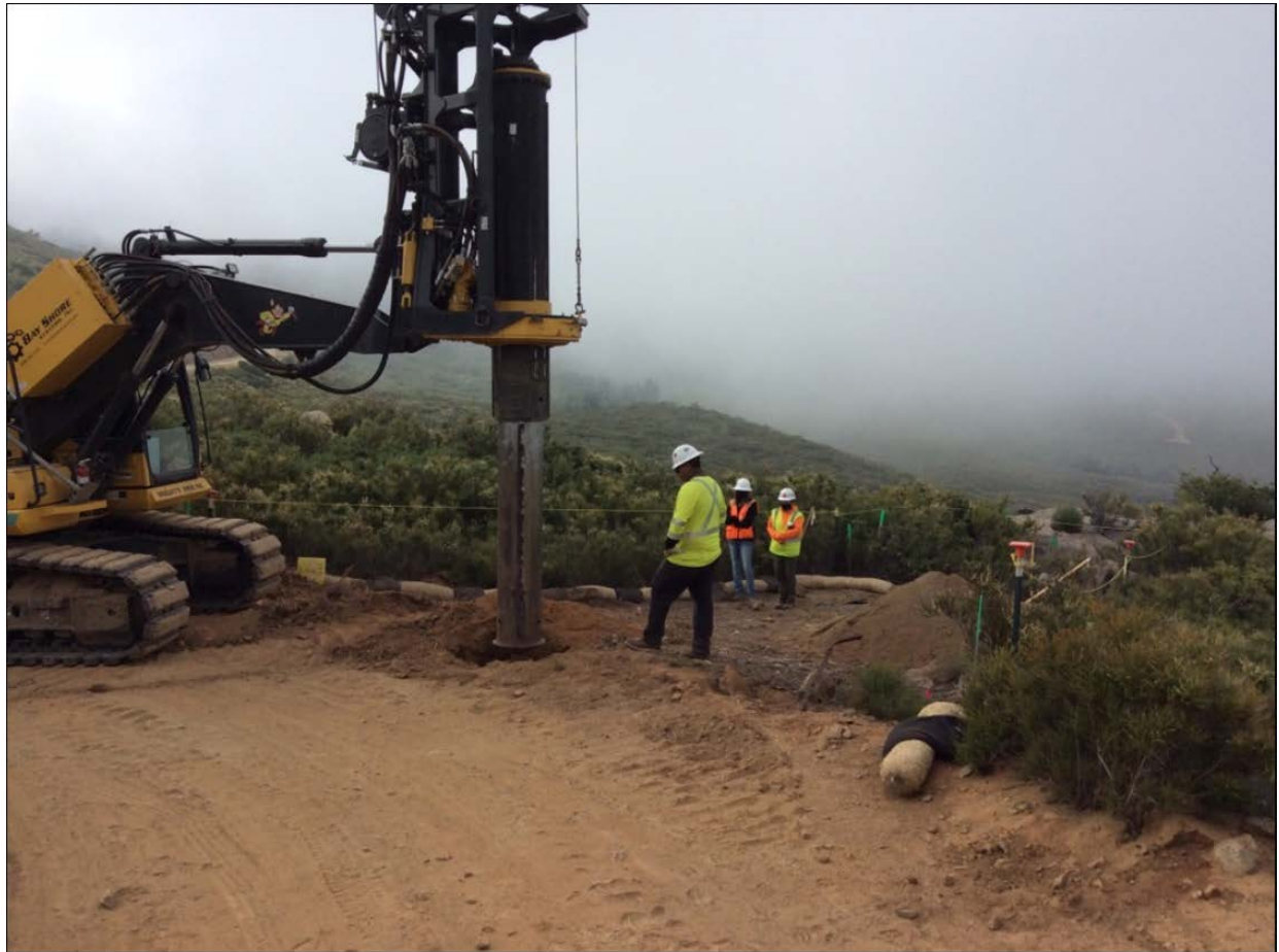
Photo 5: A crew was observed drilling a direct-bury pole hole along TL 626 Conversion South (C 79B). Archaeological and cultural monitors were observed monitoring the activity, and the surrounding ESA was clearly delineated and avoided by the crew in accordance with the HPMP (MM CUL-1), APM CUL-03, and APM CUL-04.
