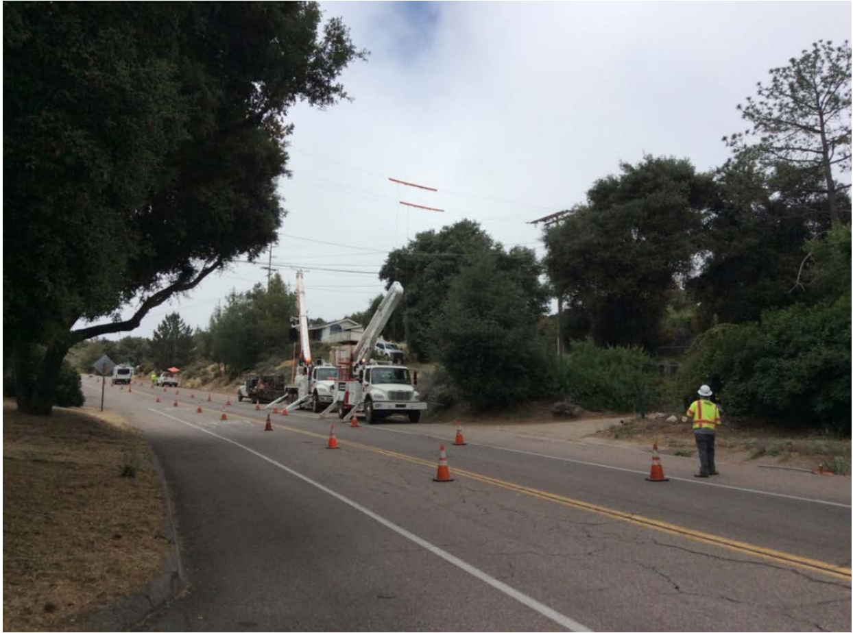
Photo 6: Cones, signage, and flagpersons were used to direct traffic through narrow lanes around the work area for P258402 and P776554 (TL 629A) in accordance with the Traffic Control Plan (APM TRANS-05) and APM TRANS-02.
