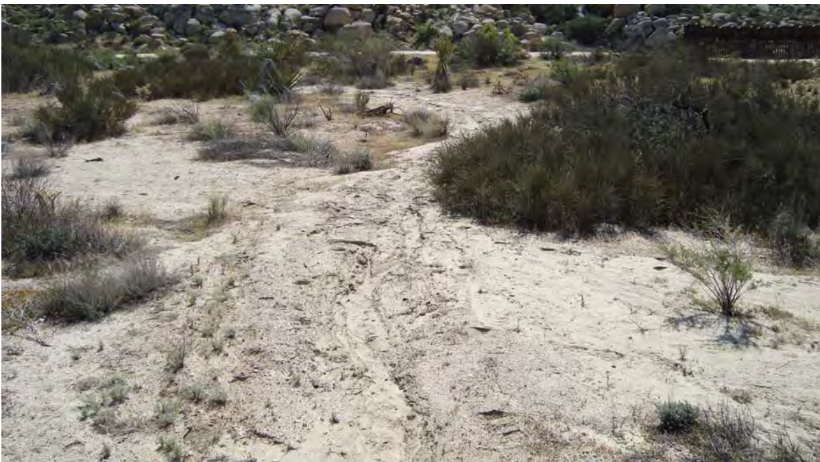
Photograph 2. View of southern erosive feature 1 looking east, with roadway in top background.
