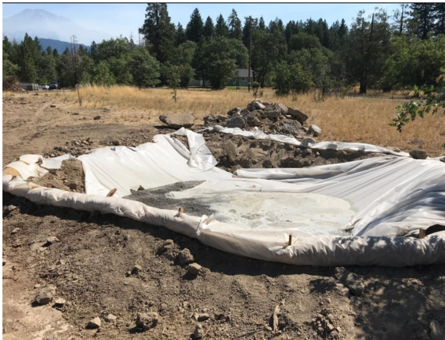
Photo 4: Concrete washout (SWPPP) liner was observed damaged and scheduled for repair.
