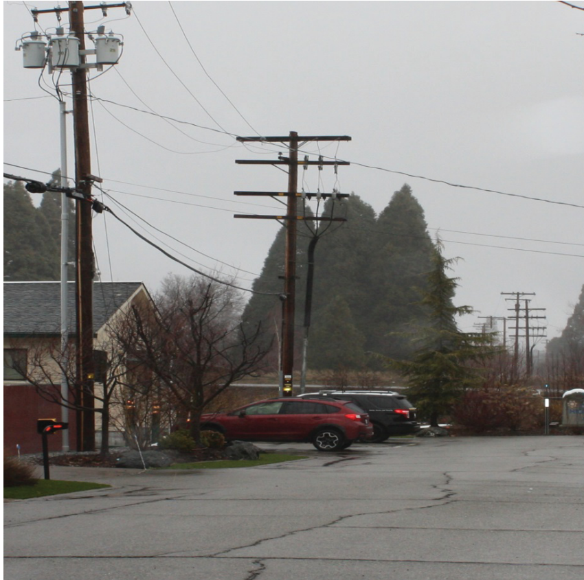
Figure 2: Existing Transmission West of I-5
